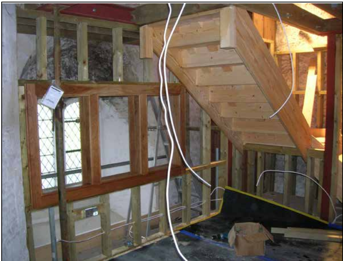
Plate 26. Office room, showing no damage caused to structure, especially to the window
