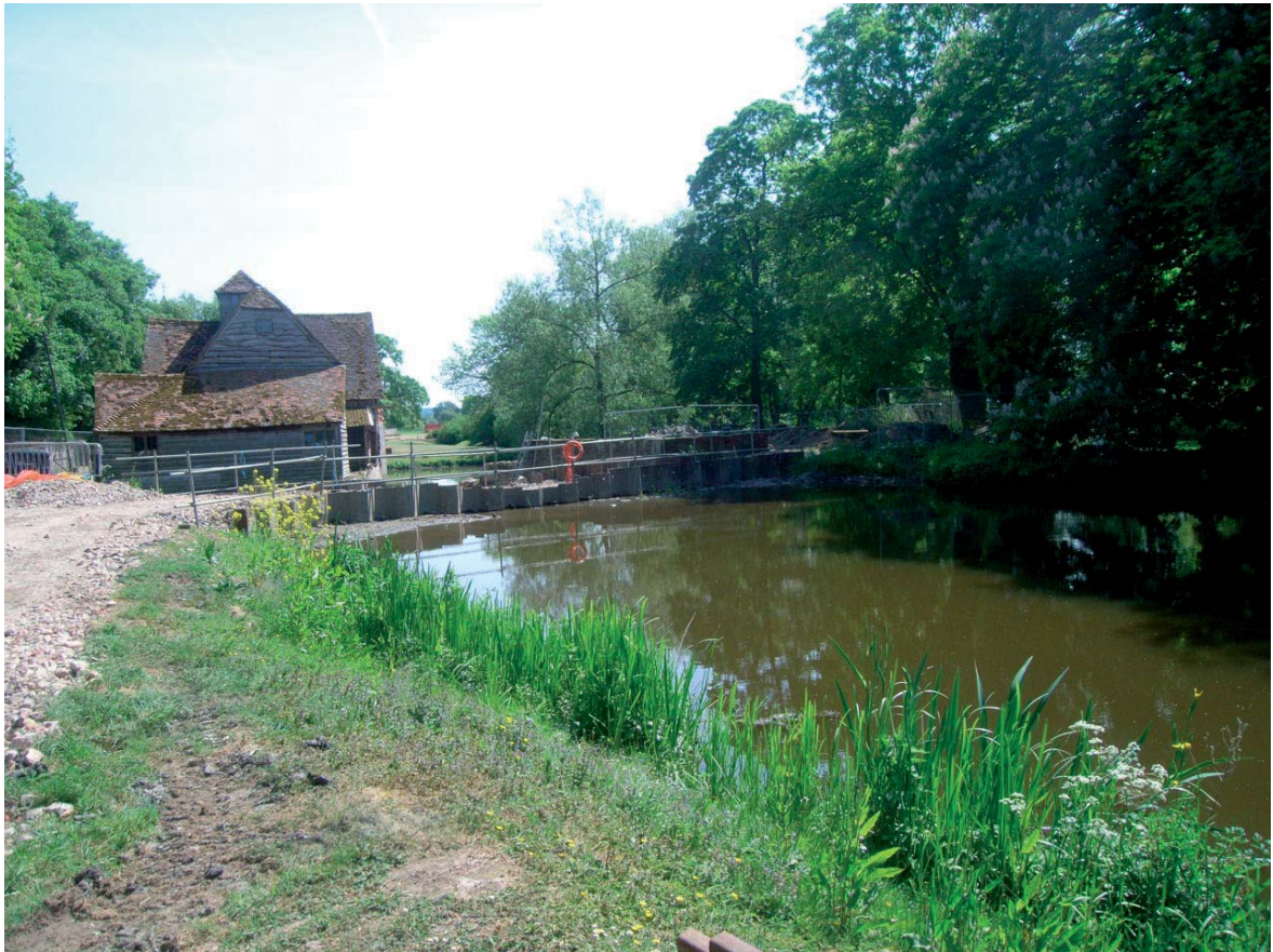
Plate 2: The temporary coffer dam and access road viewed from the west, with the mill to the rear
