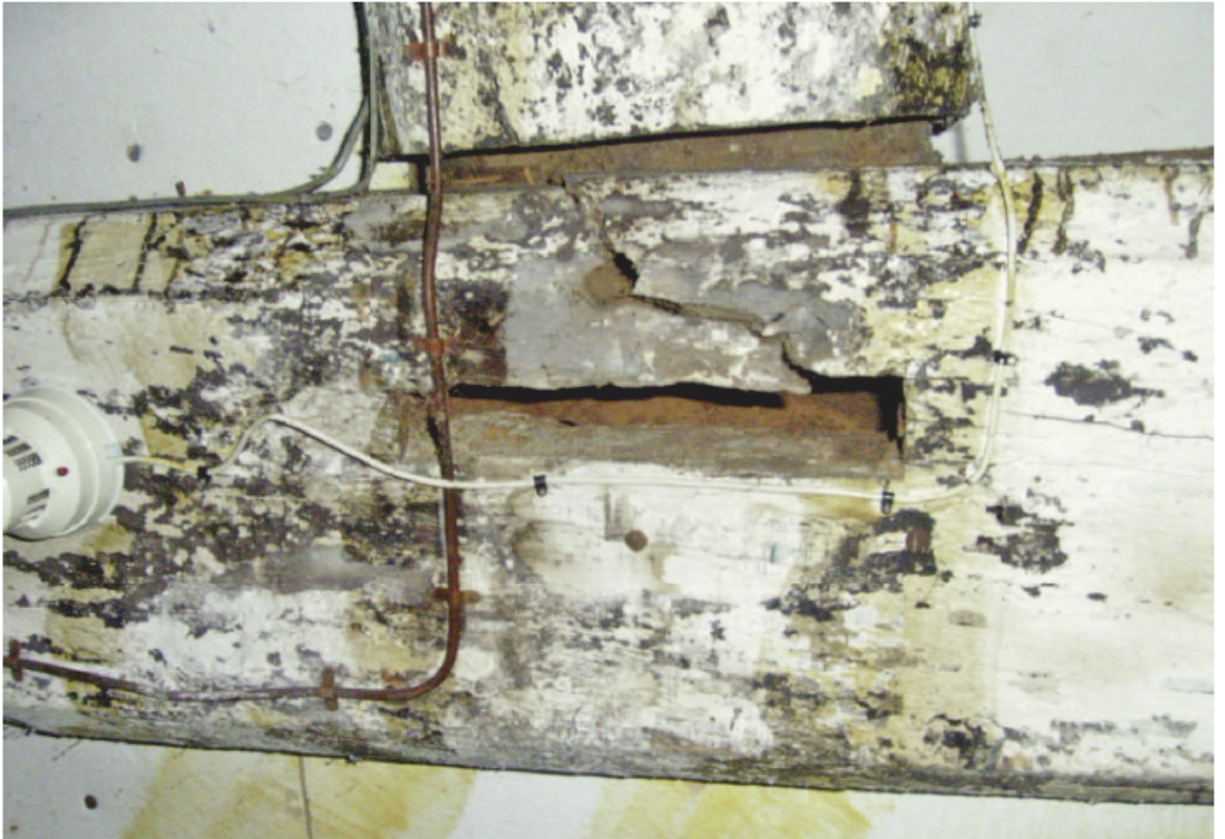
Plate 29: Tenon in Transverse Beam 12 in Area 3
