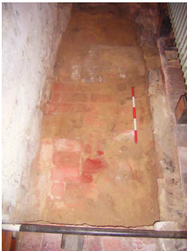
Plate 10: Exposed area of brick in south west corner of nave, facing north
