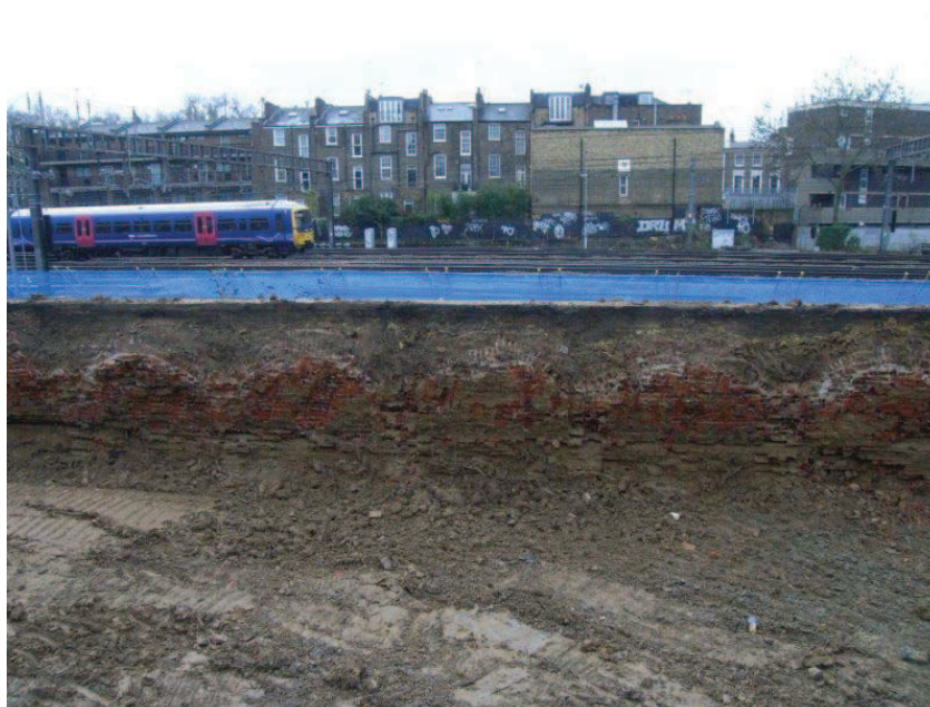
Plate 11: Arched brick structures 7025 along the southern side of the site, looking south
