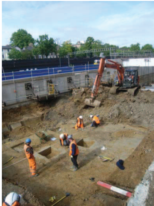
Plate 6: Manual test pitting through the lower brickearth deposits, the channel deposits and the colluvial gravels, looking south-west
