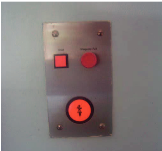
Plate 99: Alarm fitting in ground floor bedroom
