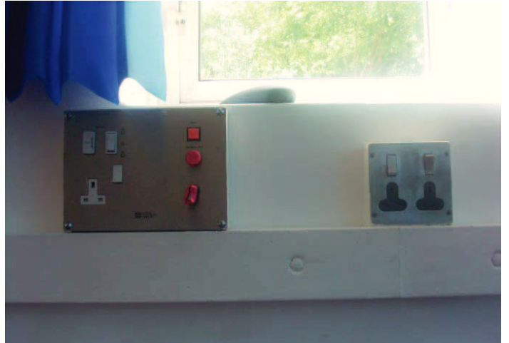
Plate 52: Wall fixtures in large treatment area in the south west wing, facing south west
