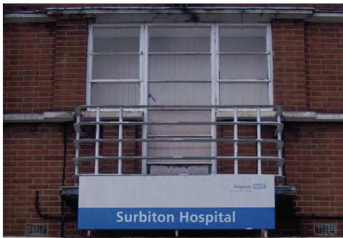
Plate 17: Detail of Juliette balcony on first floor over main entrance of hospital
