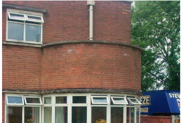
Plate 86: Protruding bay window in ground floor of south east elevation of South Bank House
