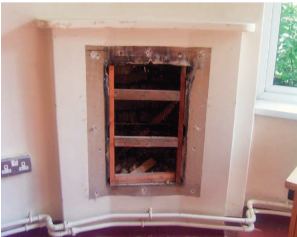
Plate 47: Unblocked fireplace in curved room at south east end of south west wing
