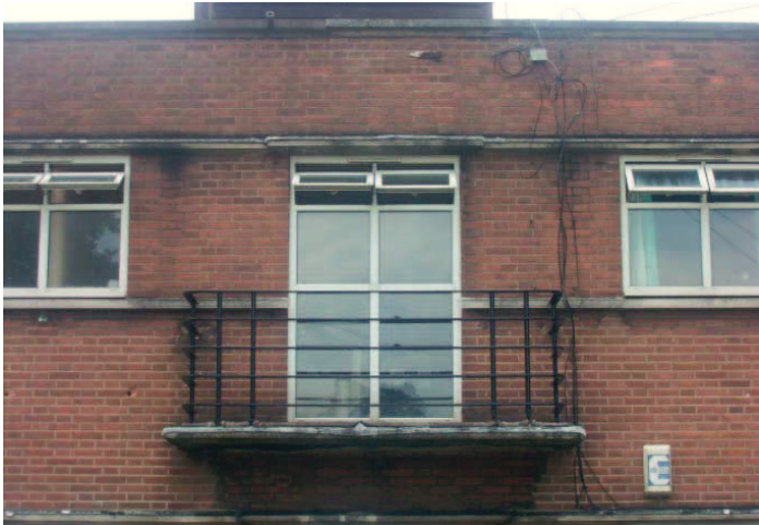
Plate 85: Balcony on first floor of south east elevation of South Bank House
