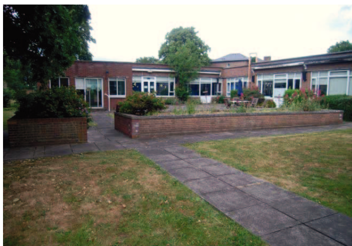
Plate 19: South west face of south west wing, viewed from south west grounds
