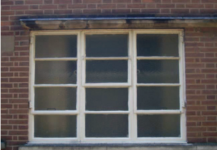
Plate 11: Primary Crittall window with central swing window and side casements on north east wing
