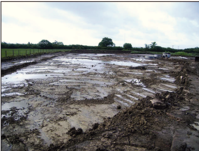
Plate 2: General view of strip, map and sample, NE side, looking SE, wet conditions
