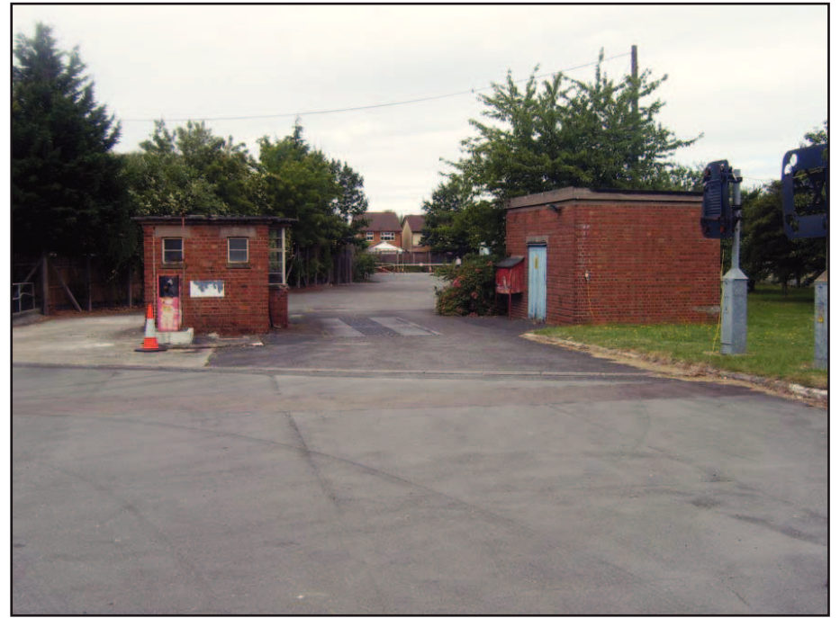
Plate 24: Electrical substation and lodge at entrance
