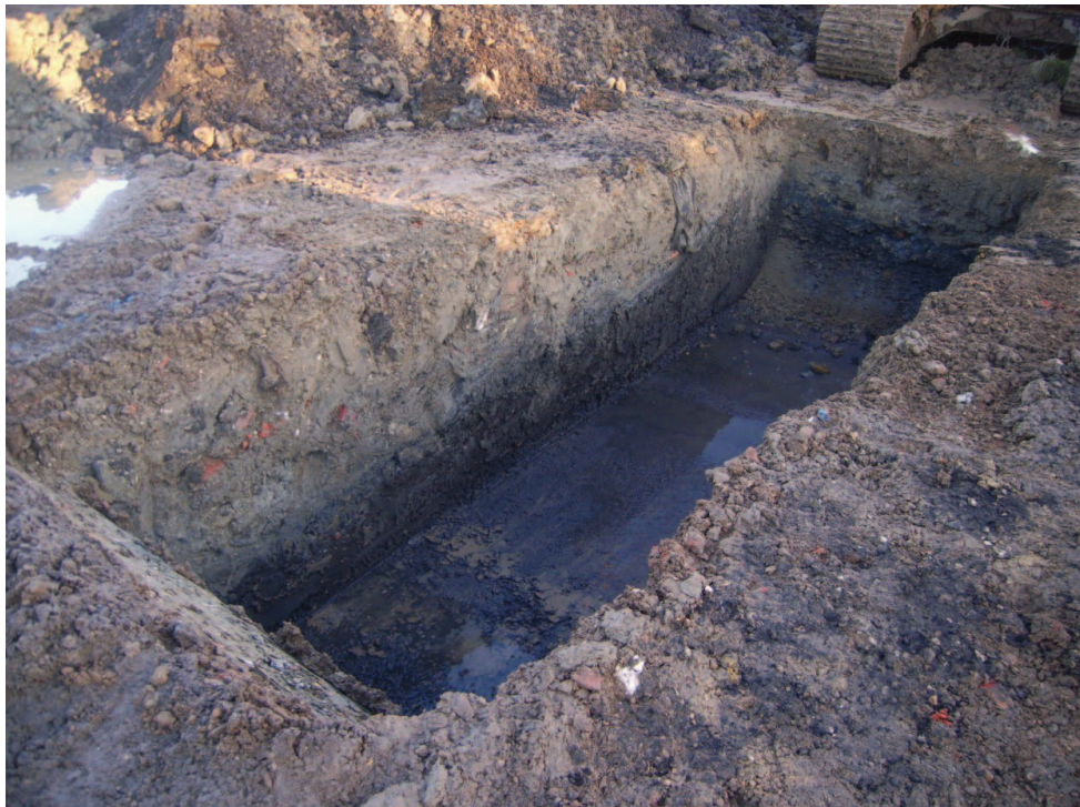
Plate 2. Oil Separator Trench; limit of excavation – the section reveals modern dumping overlying disturbed alluvial derived ploughsoil to 1.6 m below existing ground level.
