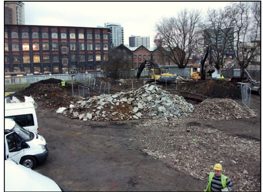
Plate 2: General View of the work area for the New Sports Hall, subject to evaluation trench mitigation looking west
