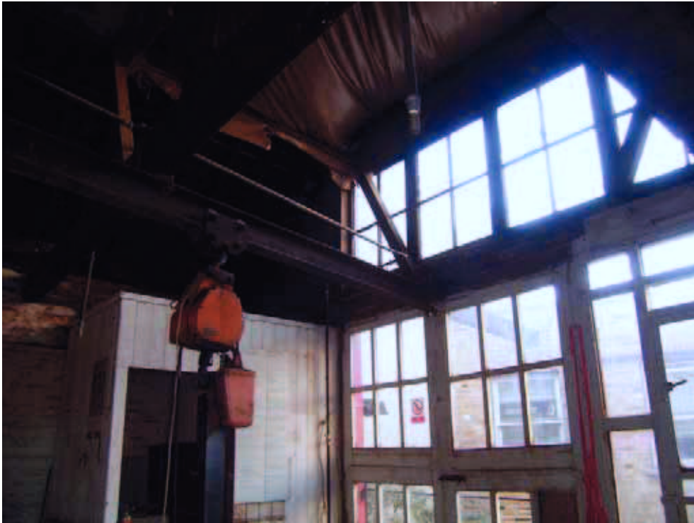
RSJ and winch attached to roof structure in north room on first floor
