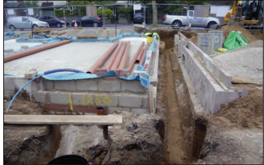
Plate 10 East – west aligned service trench between Blocks A and B (view west)
