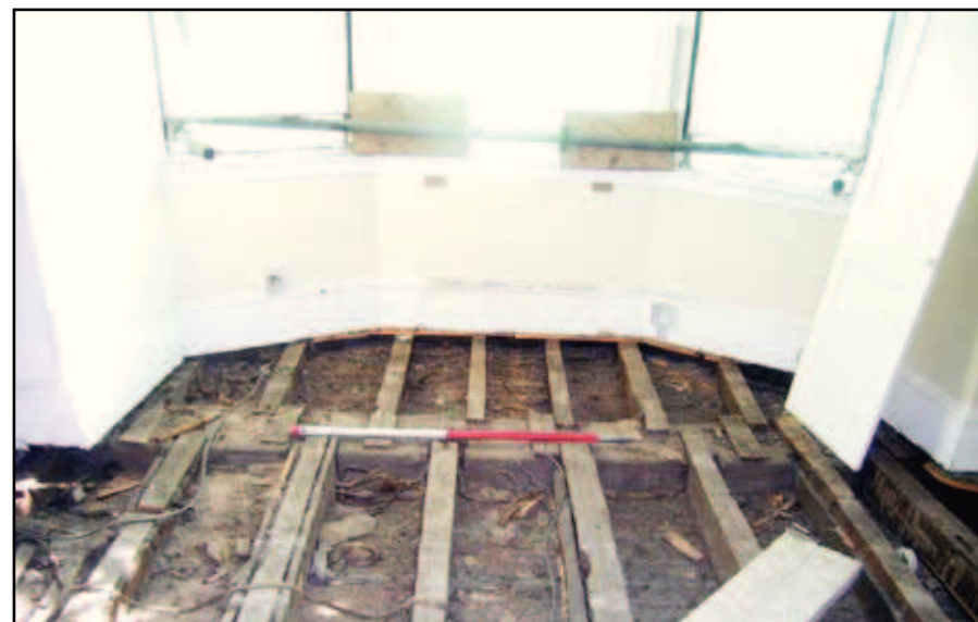
Plate 26: 27 Holywell, second floor bay window following removal of boards
