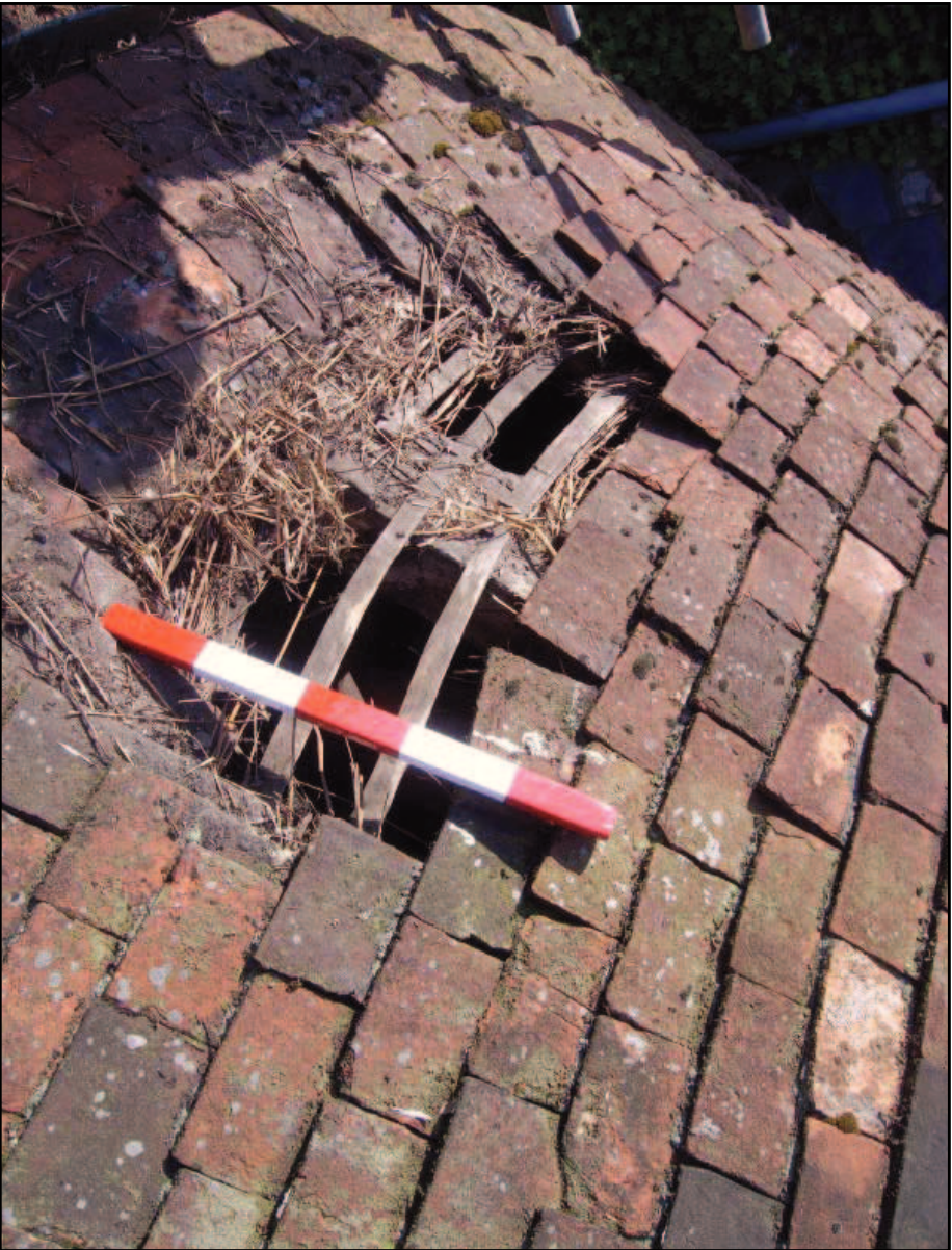
Plate 3: St. Mary's Church roof, showing straw packing
