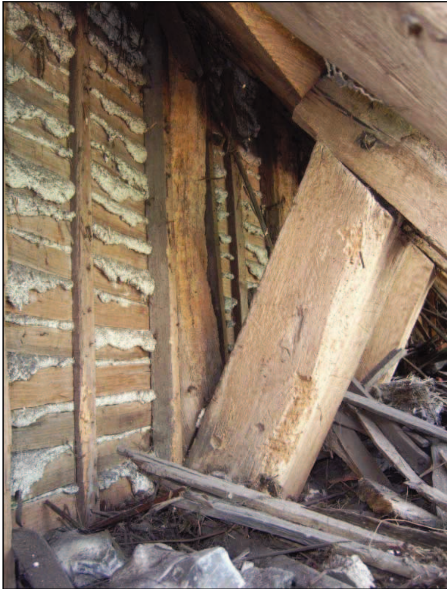
Plate 18: Strut supporting trimmer from former light
