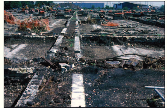
Plate 16: East view depicting brick troughs above precipitation lanes (taken during demolition works)
