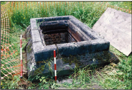
Plate 17: West view of vent above precipitation lanes
