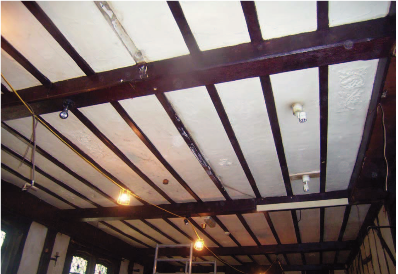
Plate 21: Ceiling in Area 3 prior to works
