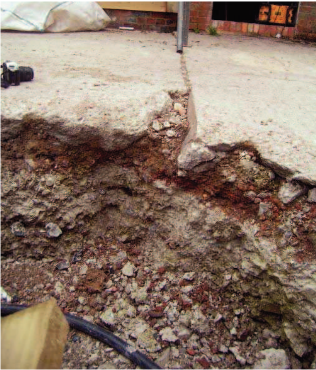
Plate 5: South side of Service Trench B immediately to north of junction between stables and medieval barn
