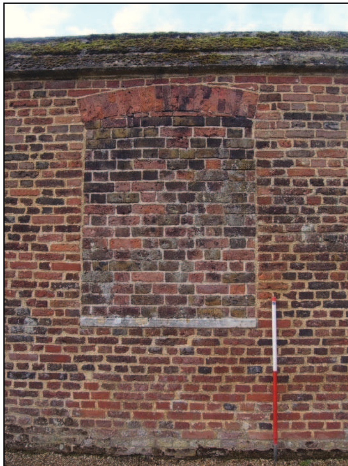
Plate 10: Infilled window opening with stone sill on north west elevation of wall
