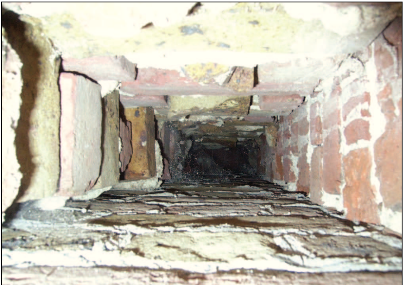
Plate 24: Internal view of void behind infill brickwork
