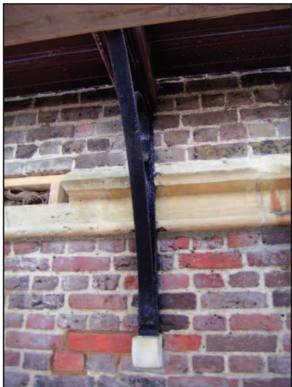
Plate 25: Iron balcony support inserted into stone string course
