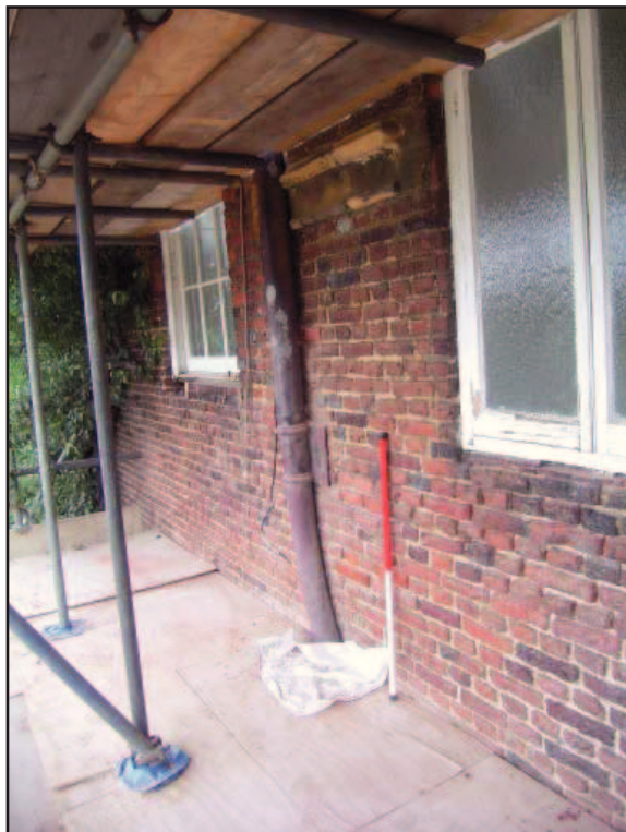
Plate 27: Inserted windows and truncated stone string course to south of tennis court range
