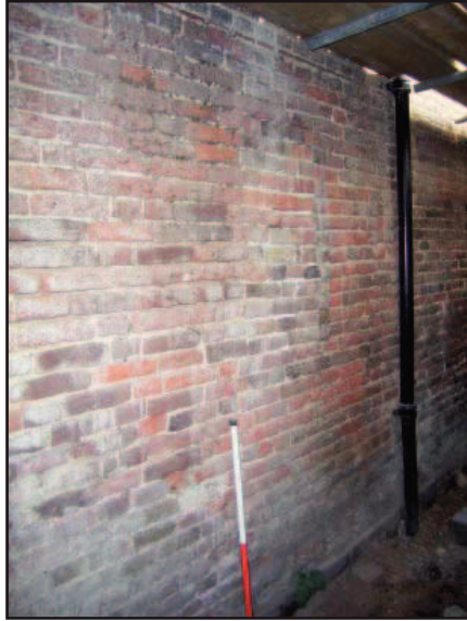
Plate 16: Infilled window opening to south end of elevation
