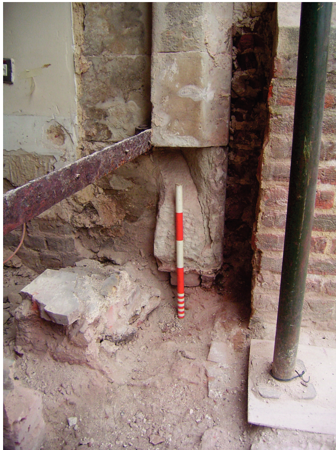
Plate 16: Detail of southwest jamb showing moulding and fractured stone
