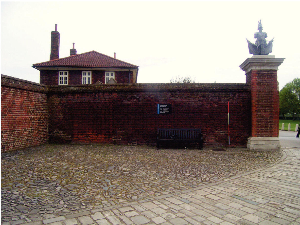
Plate 10: View of wall beside Trophy gate showing 19th and 20th century blocking in and rebuilding
