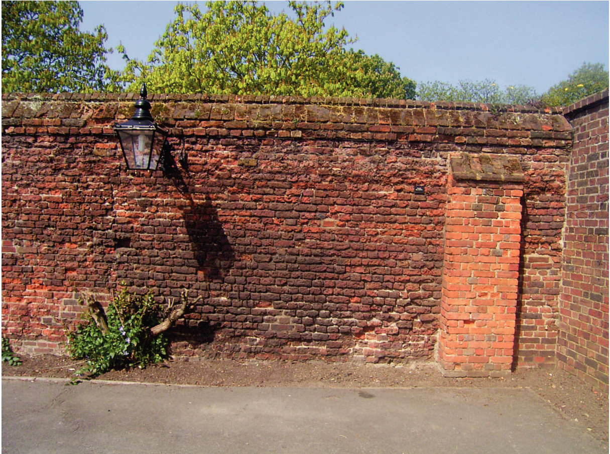
Plate 14: West elevation of west boundary wall (within car park) showing 17th century infill
