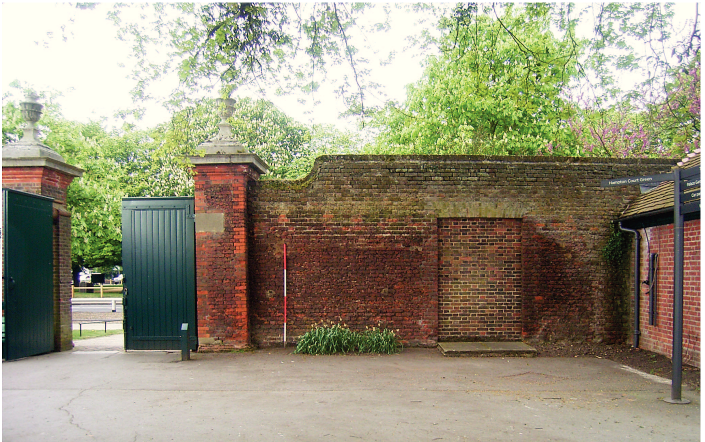
Plate 15: Gate leading onto the Vrow Walk and blocked 20th century turnstile entrance
