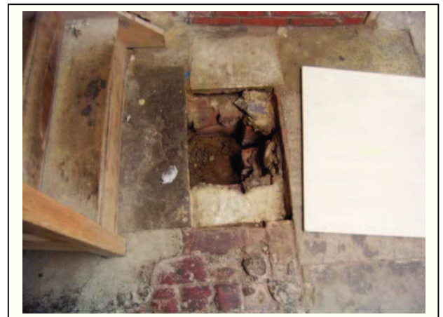
Plate 4: Raised slab in basement showing drain beneath.
