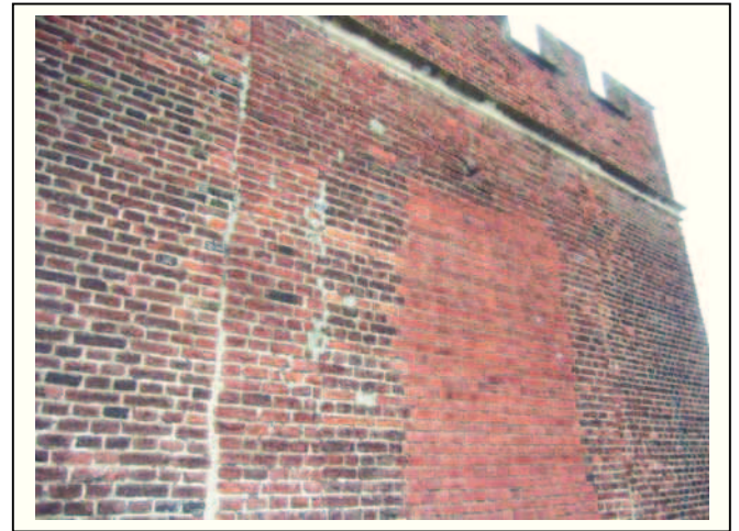
Plate 2: Blocked features on the south wall investigation focused on the area above the large blocked window.
