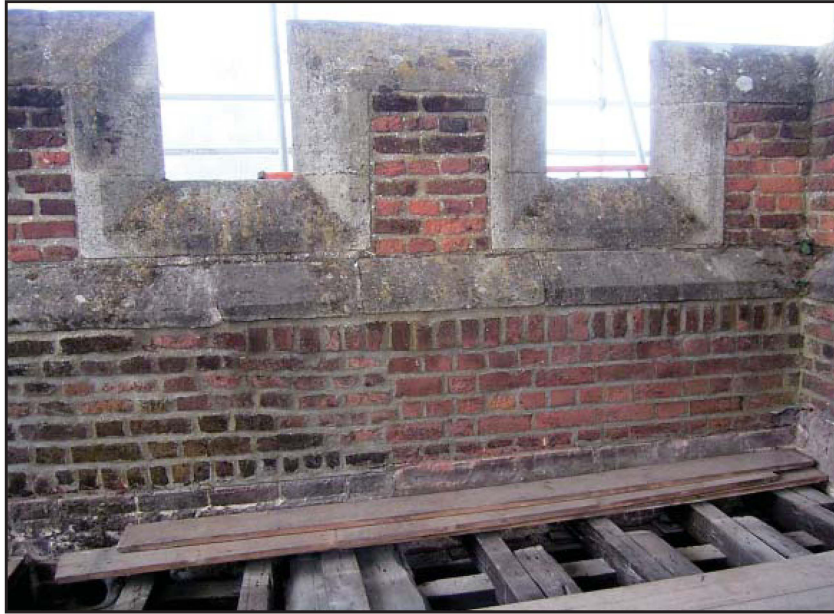
Plate 48: West parapet, internal face, showing 20th century rebuild (to right of picture)
