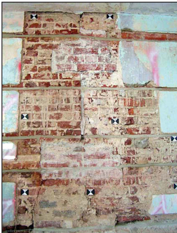
Plate 58: South elevation, first floor, internal view, showing 19th and 20th century patching
