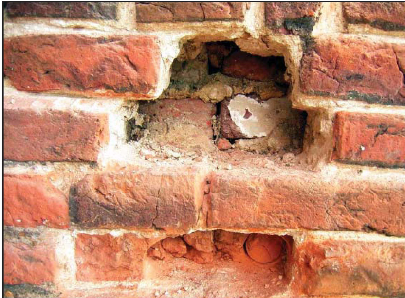
Plate 36: North elevation, second floor, exposed brickwork during brick replacement, illustrating reclaimed bricks on second skin
