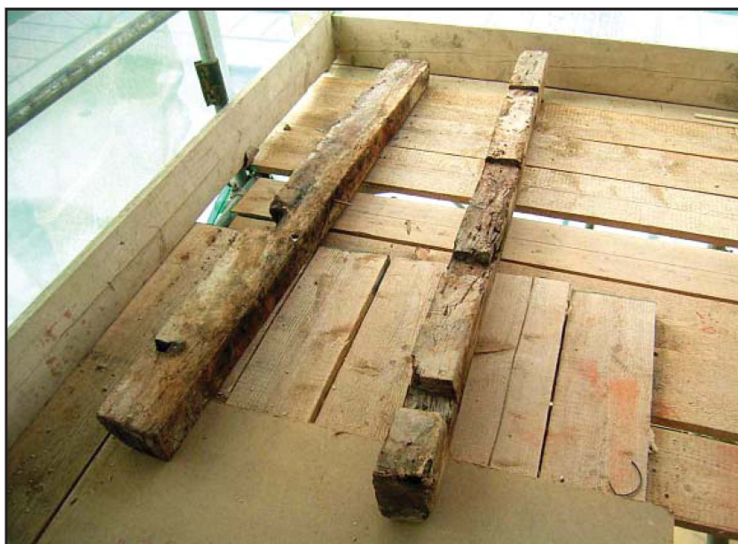
Plate 55: West elevation, illustrating two removed timber lintels exposed above second floor window
