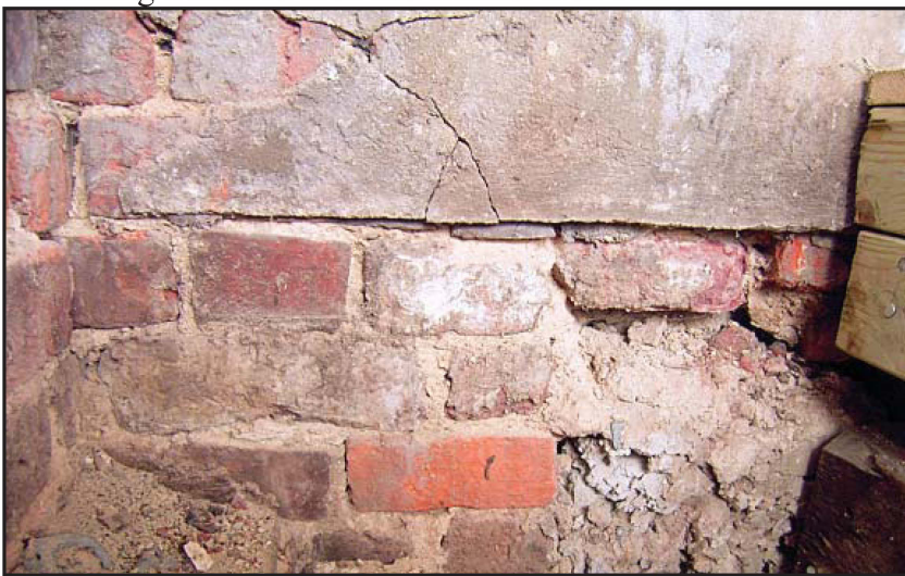
Plate 34: North elevation, north-west corner of parapet, infilled outlet/drain
