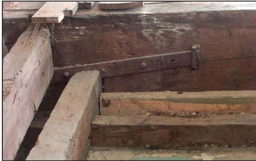
Plate 57: Parapet floor, south view illustrating iron strap secured on truss
