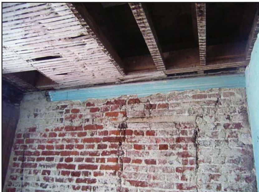
Plate 61: East elevation, internal view, second floor, pipe exposed below ceiling
