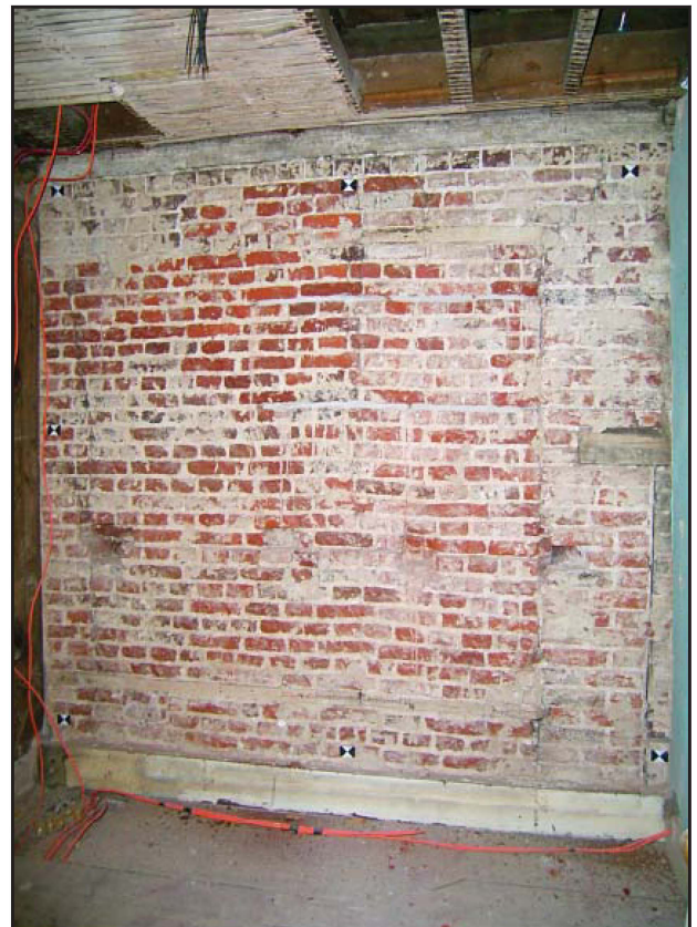
Plate 5: East elevation, internal view, second floor, illustrating vertical Tudor break to south
