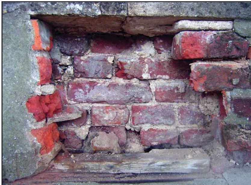
Plate 40: East parapet, internal face, showing inner Tudor core
