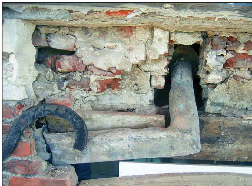
Plate 54: West elevation, external view, second floor, illustrating lead pipe squashed behind brick
