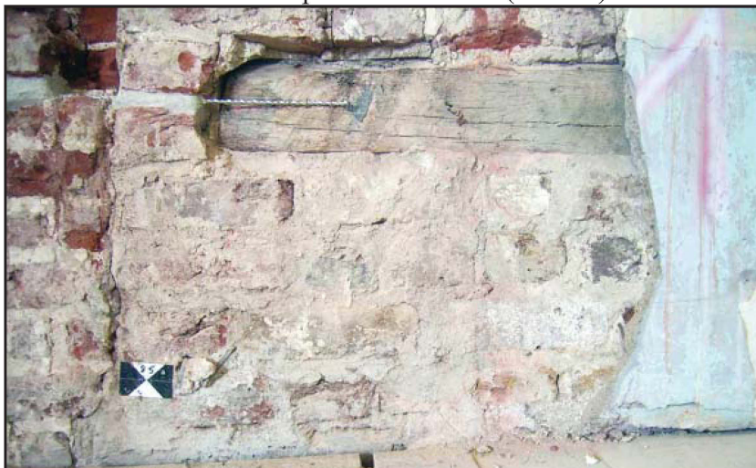
Plate 26: South elevation, internal view, first floor, showing timber lintel at base of exposed brickwork (to east)
