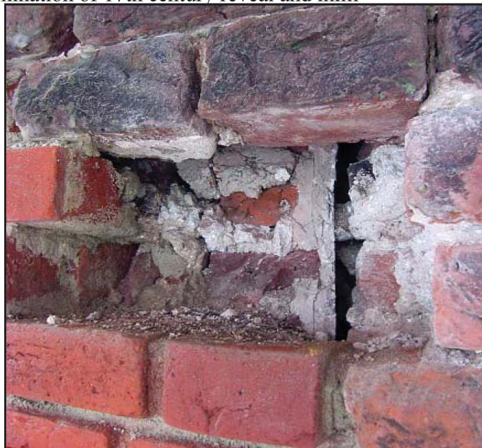
Plate 24: South elevation, external view, second floor, showing 17th century window reveal identified during brick replacement
