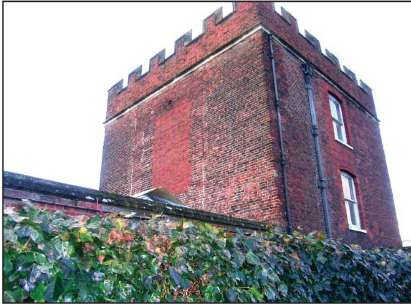
Plate 3: South (and east) elevation, showing central panel of infill and location of former window (pre-works)
