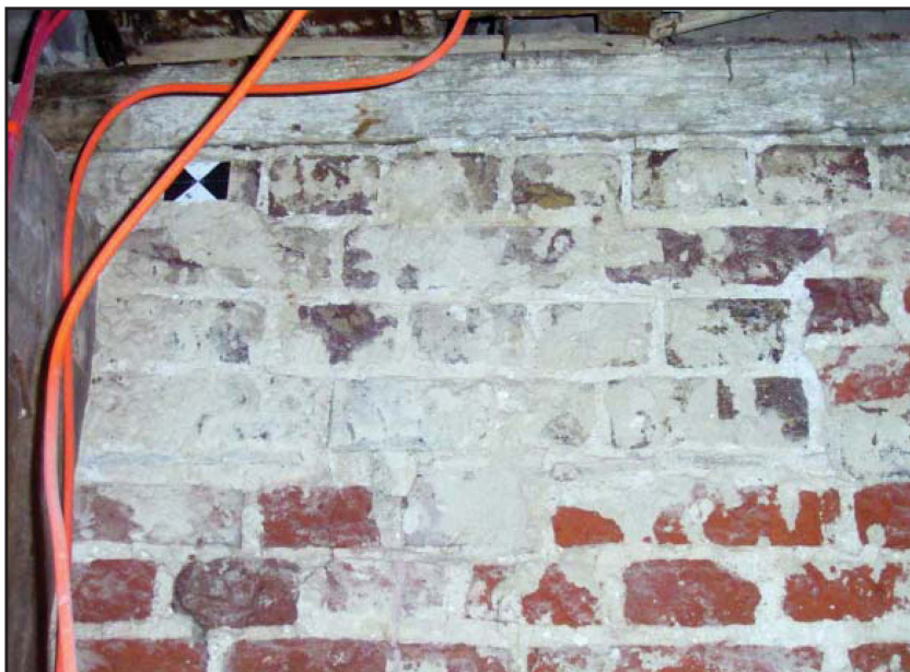
Plate 38: East elevation, second floor, internal view, showing late 17th - early 18th bricks used to level off below ceiling level
