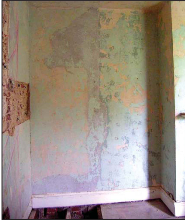
Plate 62: Internal west wall, first floor level, illustrating wall scar from dumb waiter
