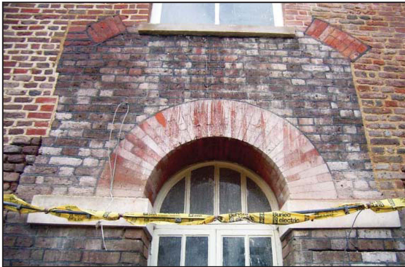
Plate 33: East elevation, external view, ground and first floors, illustrating truncated arch and strainer arch below
