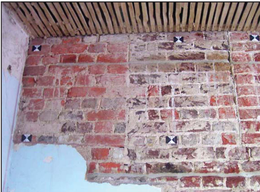
Plate 23: South elevation, internal view, first floor, showing termination of 17th century reveal and infill
