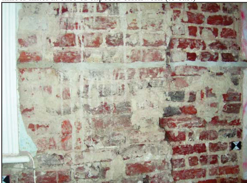
Plate 27: East elevation, internal view, second floor, showing two infilled joist pockets (to right of picture)
