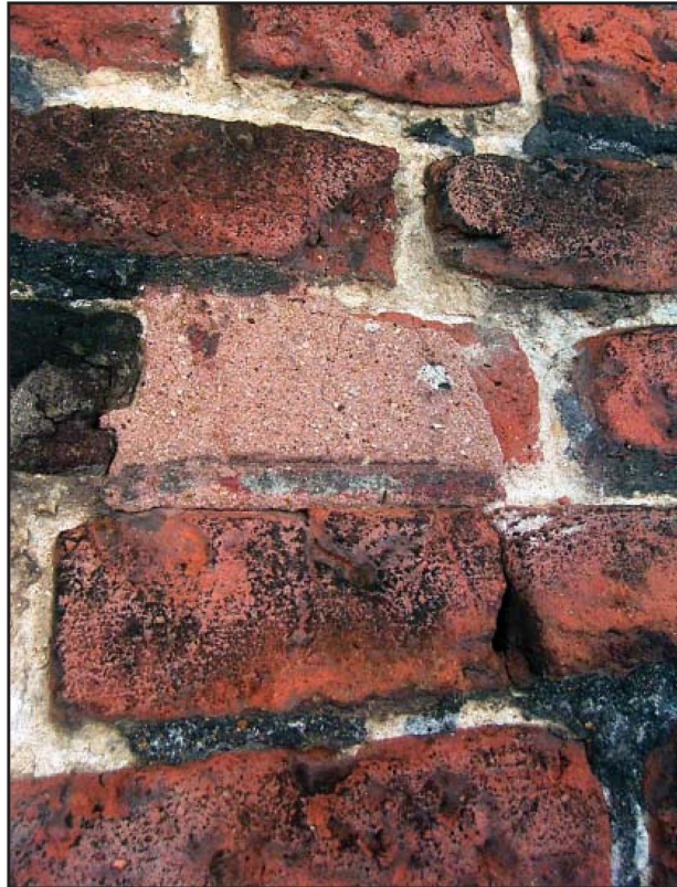
Plate 65: West elevation, ground floor, external view, illustrating repair to bricks and penny roll pointing
