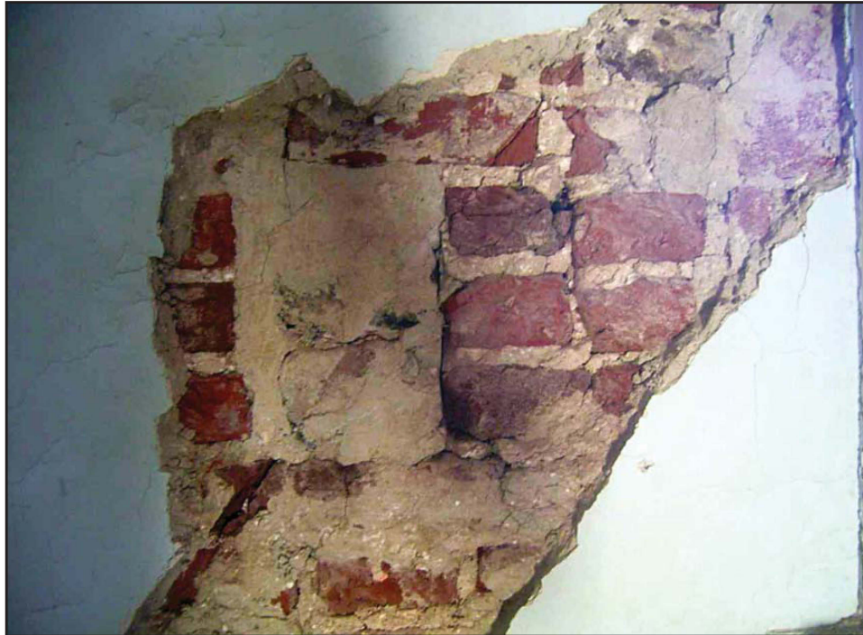
Plate 28: West elevation, internal view, first floor, showing infilled joist pocket to south of window
