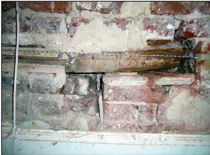
Plate 22: East elevation, internal view, first floor, illustrating timber lintel and north reveal
