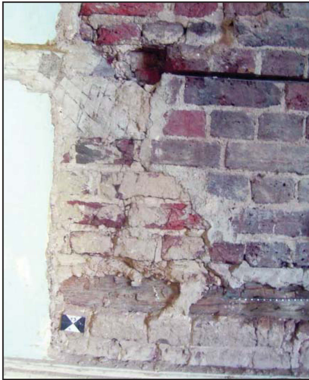
Plate 25: South elevation, internal view, first floor, showing timber lintel at base of exposed brickwork (to west)
