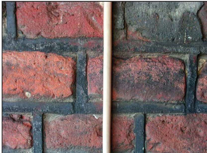
Plate 66: West elevation, first floor, external view, illustrating red paint on black ash pointing
