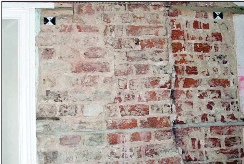
Plate 51: East elevation, internal view, illustrating 1888-1924 brickwork to south of window (and Phase 3 and 2 further to right of picture)
