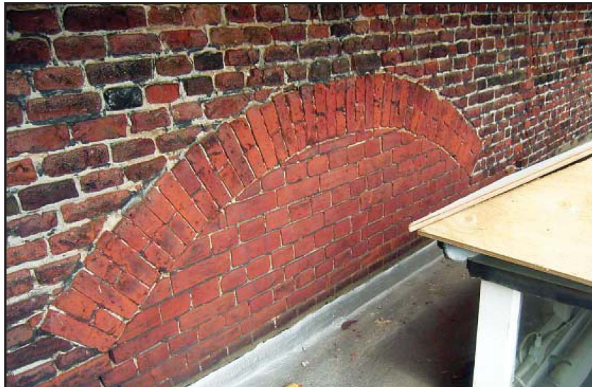
Plate 32: South elevation, external view, ground floor, late 17th - early 18th century arch
