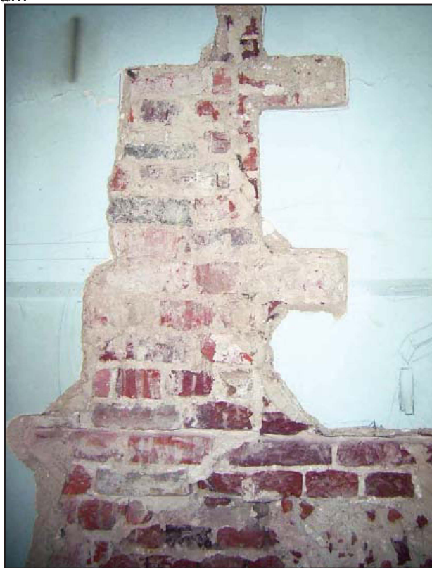
Plate 35: North elevation, first floor, internal view, illustrating salvaged bricks at top of exposed brickwork
