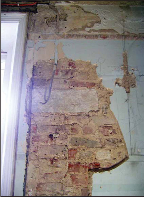
Plate 59: West elevation, first floor, internal view, showing stone within 17th century area of rebuild
