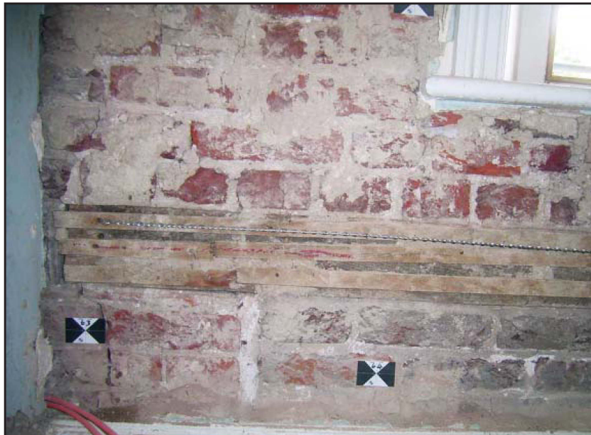
Plate 21: East elevation, internal view, first floor, illustrating timber lintel and south reveal
