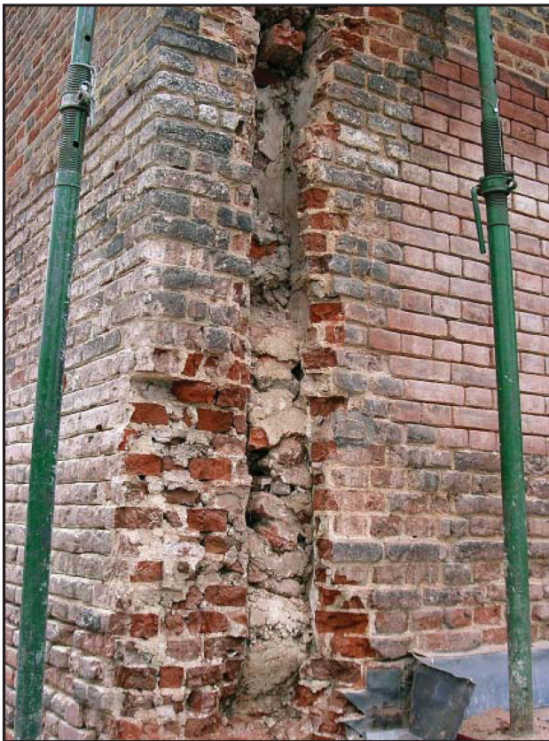
Plate 13: West elevation, external view, showing vertical shaft during removal of rubble infill
