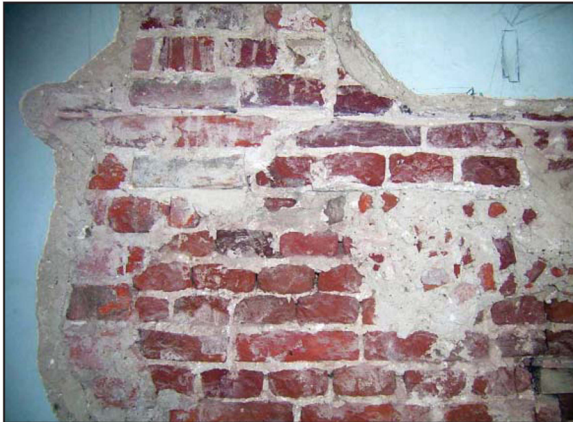
Plate 37: North elevation, first floor, internal view, illustrating surviving Tudor bricks to base of exposed brickwork
