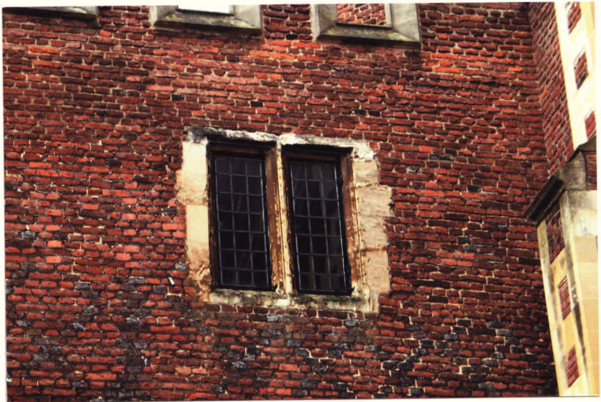
Plate 4. Clock Court, north-west corner 2nd floor window with Beer stone lintel & Bath stone jambs and sill.
