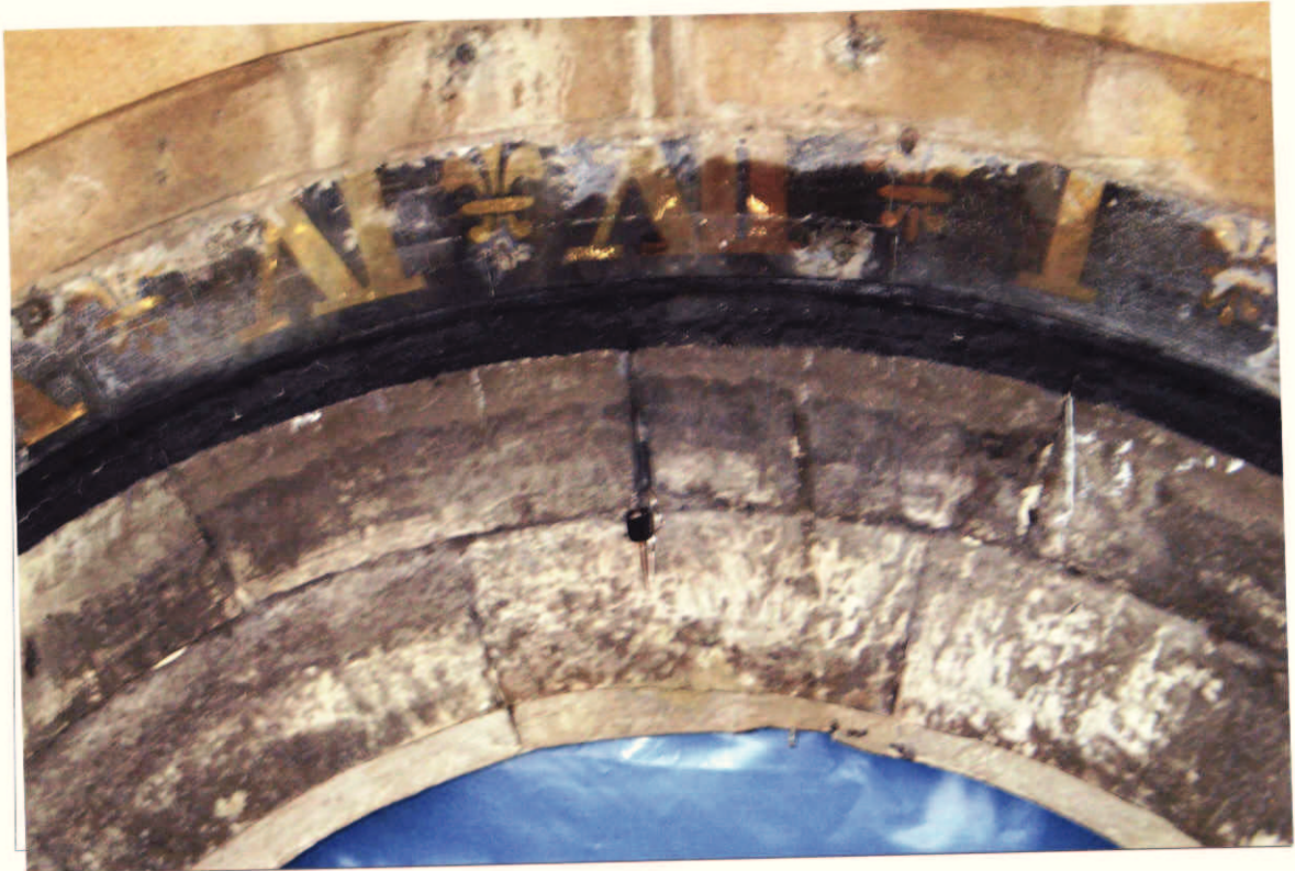
Plate 7. Detail of Plate 6. The yellow outer stone of the surround is a 20th century Clipsham stone restoration.
