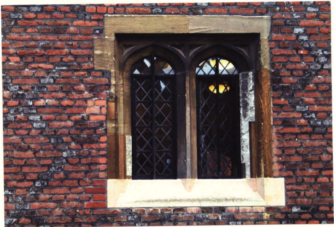
Plate 3. Base Court, ground floor window showing four phases of construction and repair. In order - Reigate stone (grey), Wheatley Limestone (grey-brown), Bath stone (brown), 20th century Bath Stoke Ground Base Bed (sill).
