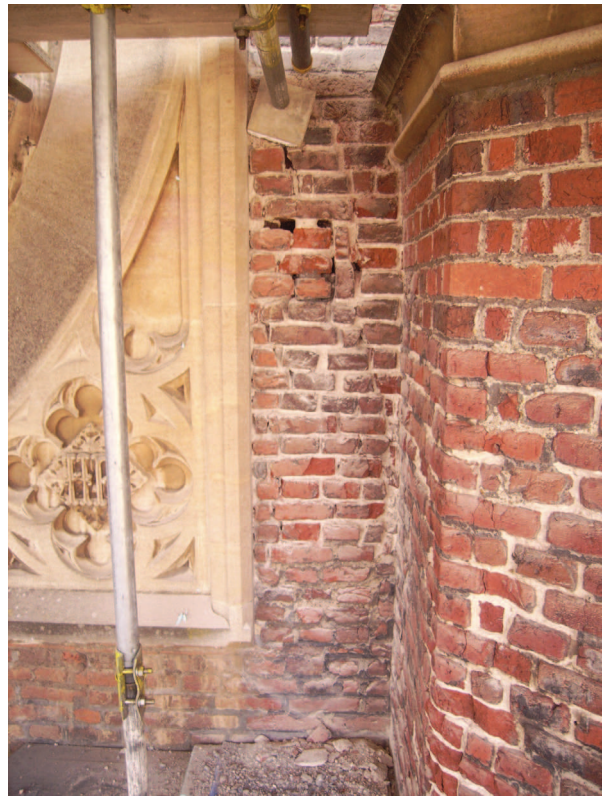
Plate 13: Putlog beside Astronomical clock stonework
