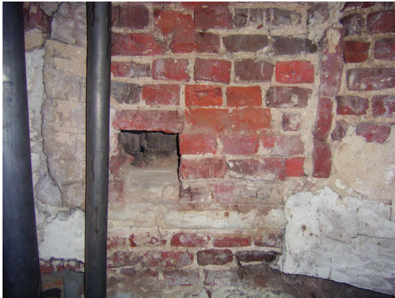
Plate 21: SW turret interior, blocked window
