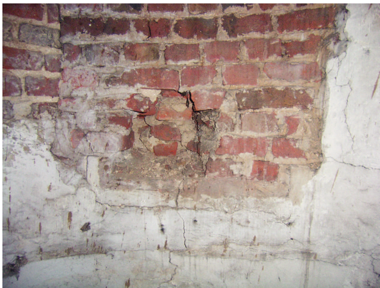
Plate 22: SW turret interior, blocked window
