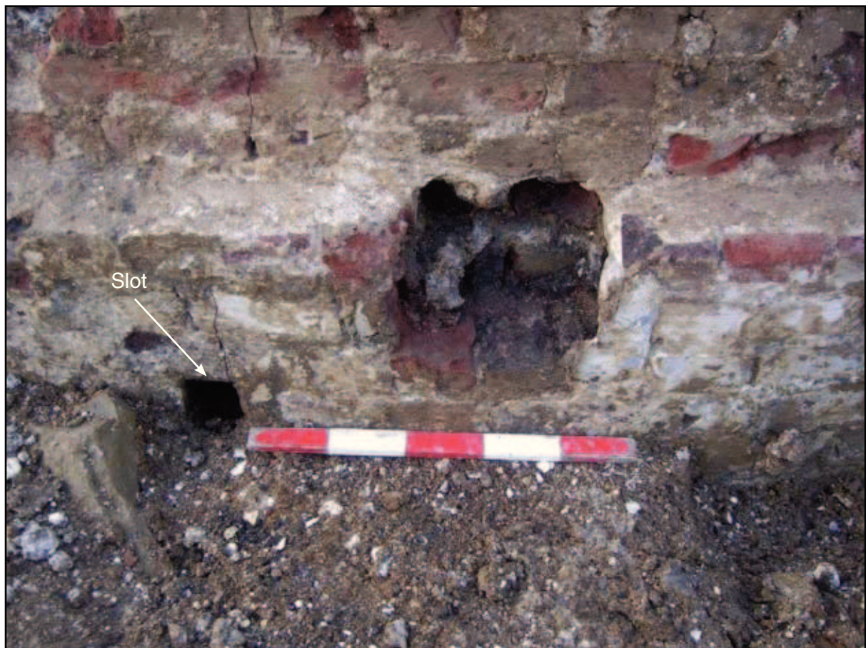
Plate 4: Trench 2. Elevation view of recess for horizontal support in wall 3001, and window slot visible, looking north-west
