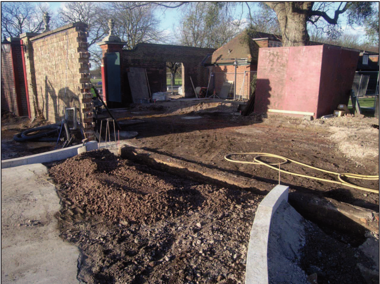
Plate 2 - View through the break in the 19th century garden wall toward Vrow Walk Gate during the groundwork. Upper Car Park (Area H) is the left and the walkway
