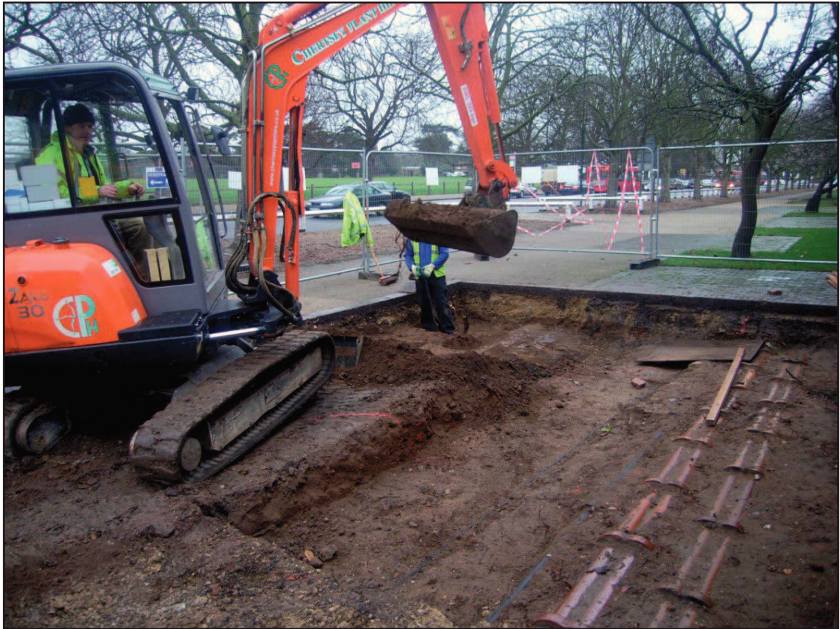
Plate 1 - Machine excavation in Area C exposing modern services . The roadside verge (Area A) and Vrow Walk (Area B) can be seen in the background
