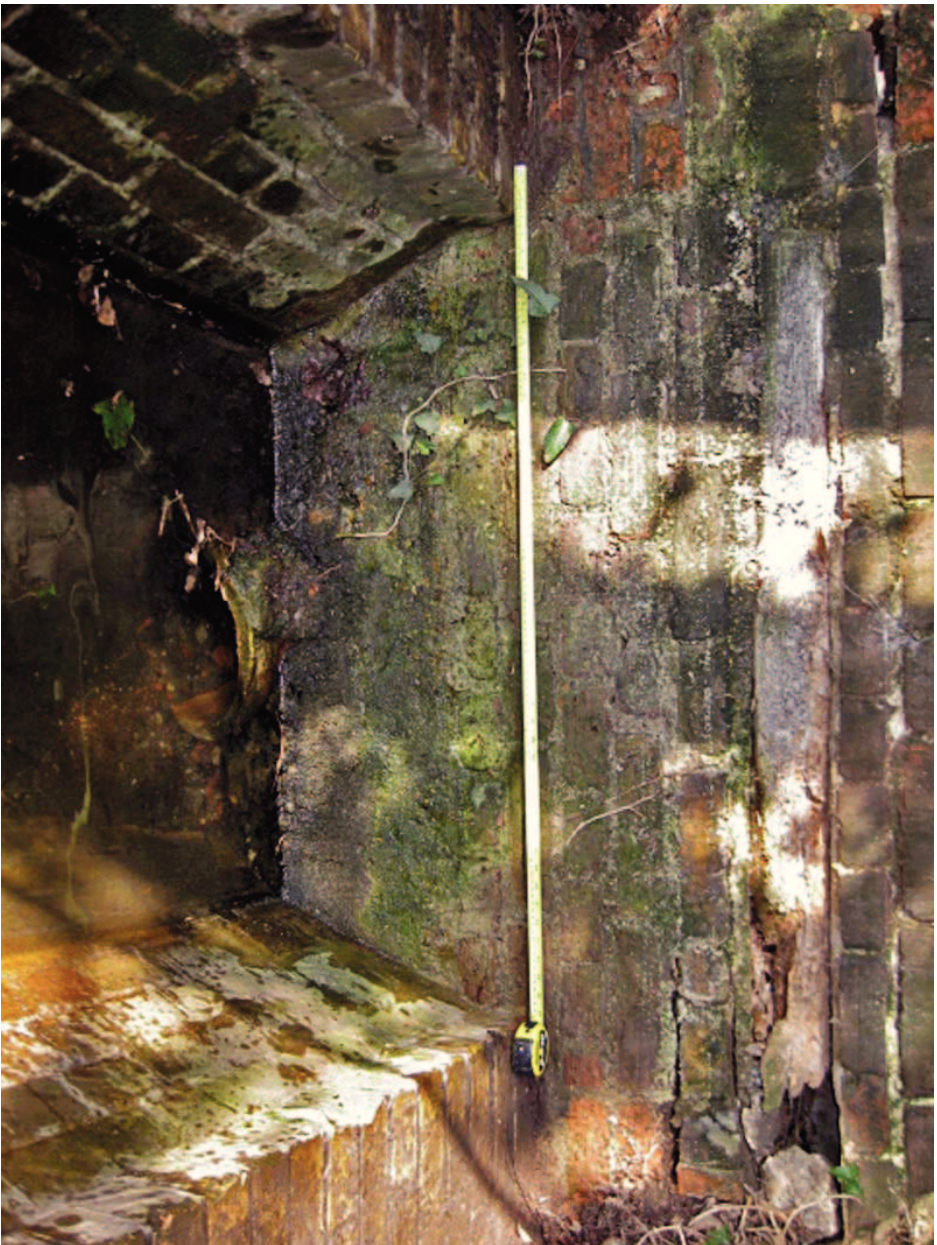
Plate 2: Detail of water inlet, looking north
