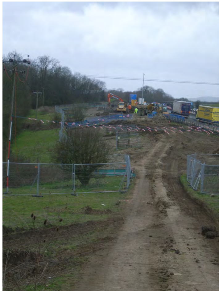
Figure 5: General view of the construction and excavation area showing the motorway embankment. View west
