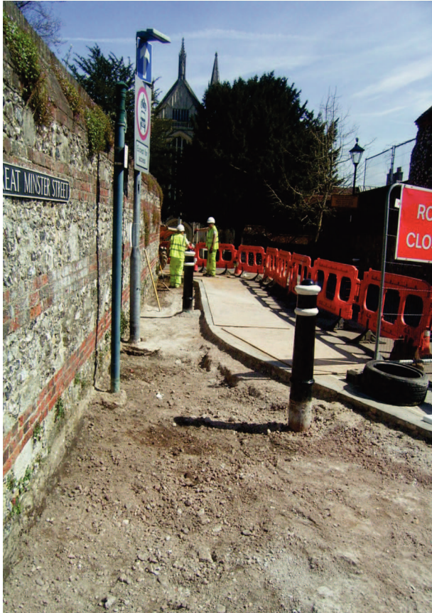
Plate 1: Pavement (at junction with Little Minster Street) at formation level - looking E
