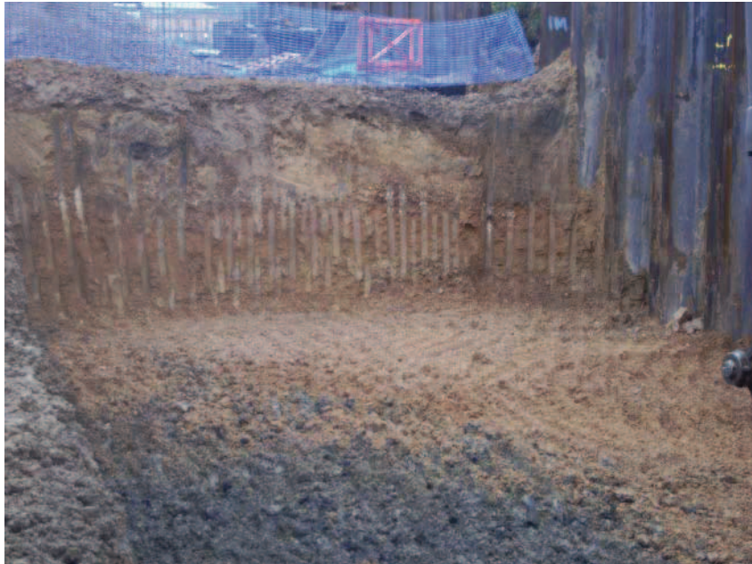
Plate 2: Made ground, 'undisturbed' layers and gravels in section from original ground level
