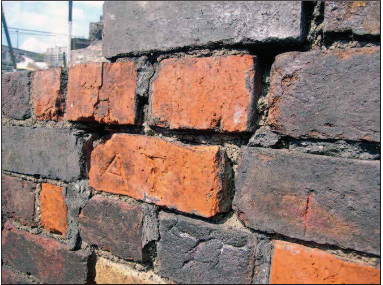
Plate 9: Graffiti on northern wall of engine house [8528]
