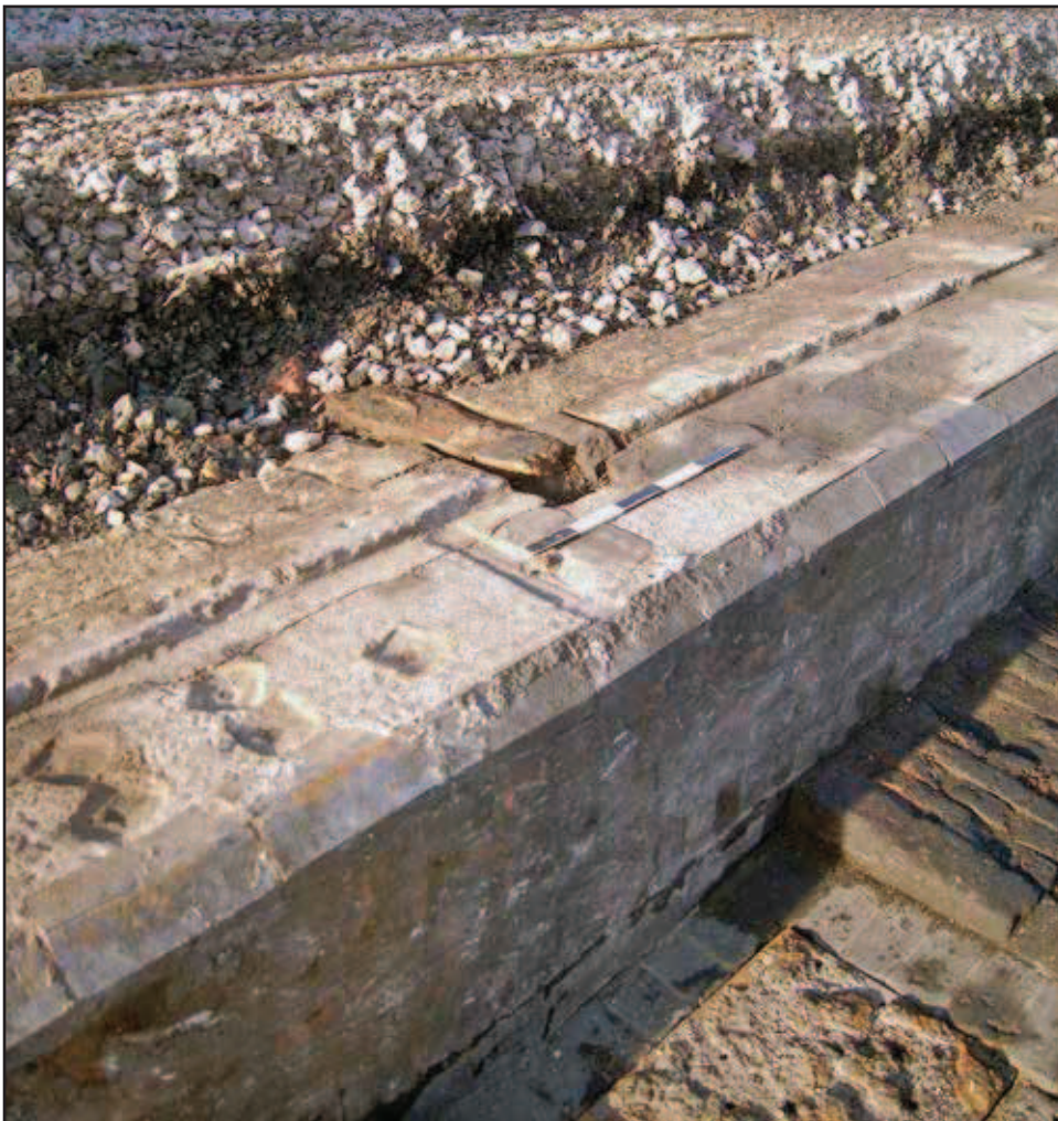
Plate 52: Detail of standard gauge pit wall showing timber sleeper and marks of screw jacks
