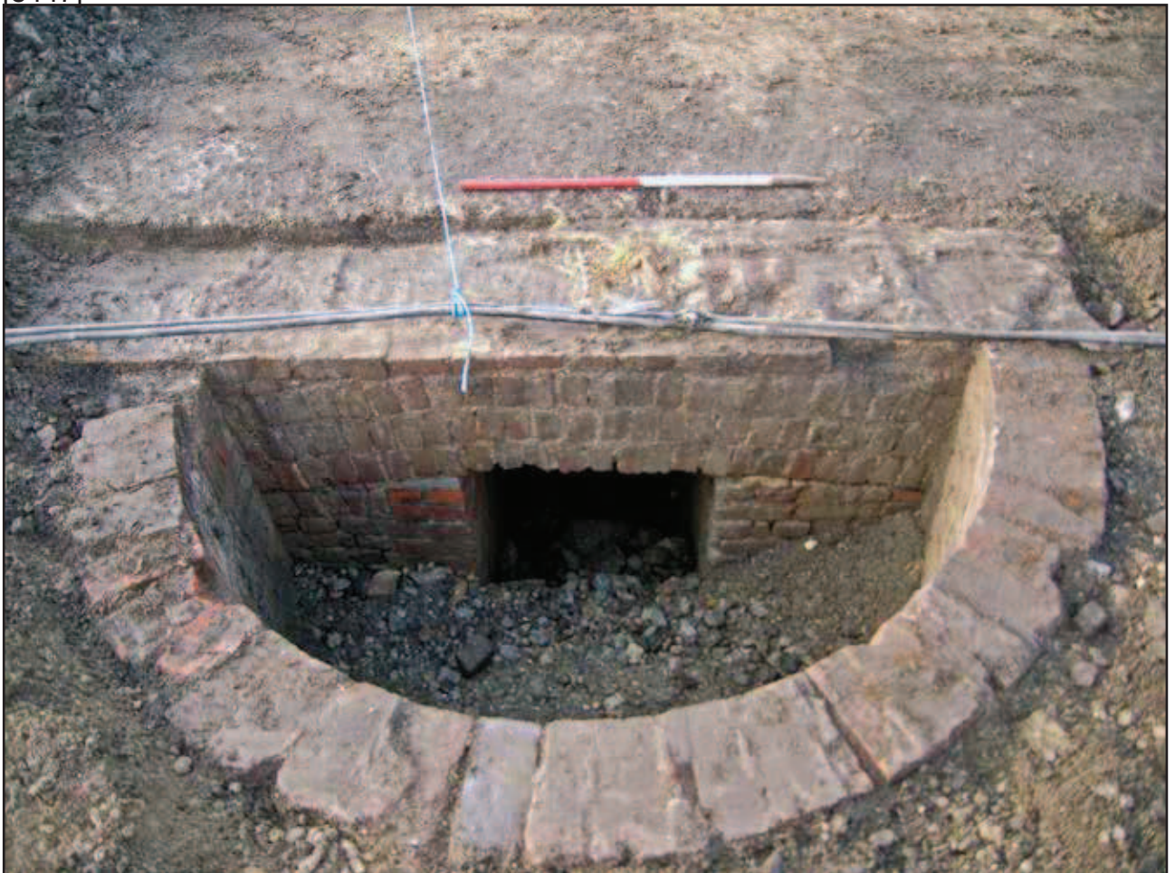
Plate 54: Semi circular inspection chamber [8854] into Marcon Sewer added to outside of northern wall of Broad gauge shed
