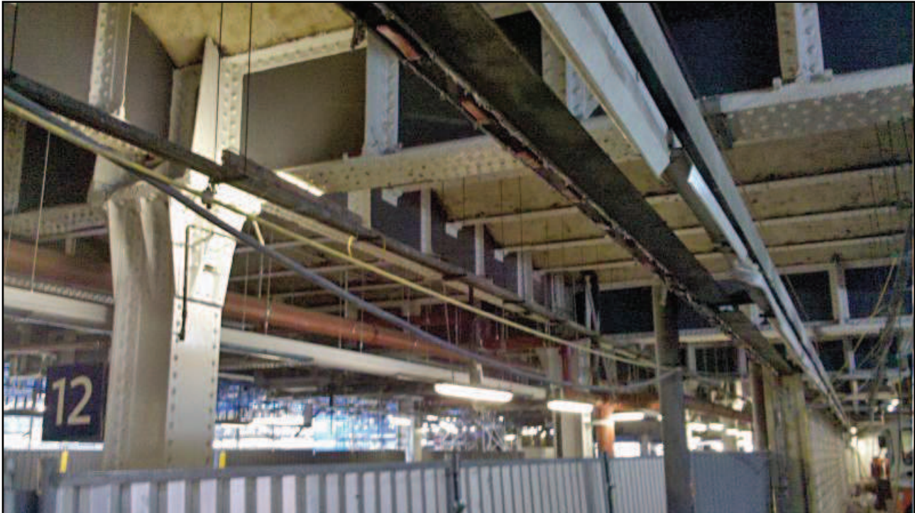
Plate 22: Continuation of the same iron ceiling and support structures on Platforms 11 and 10
