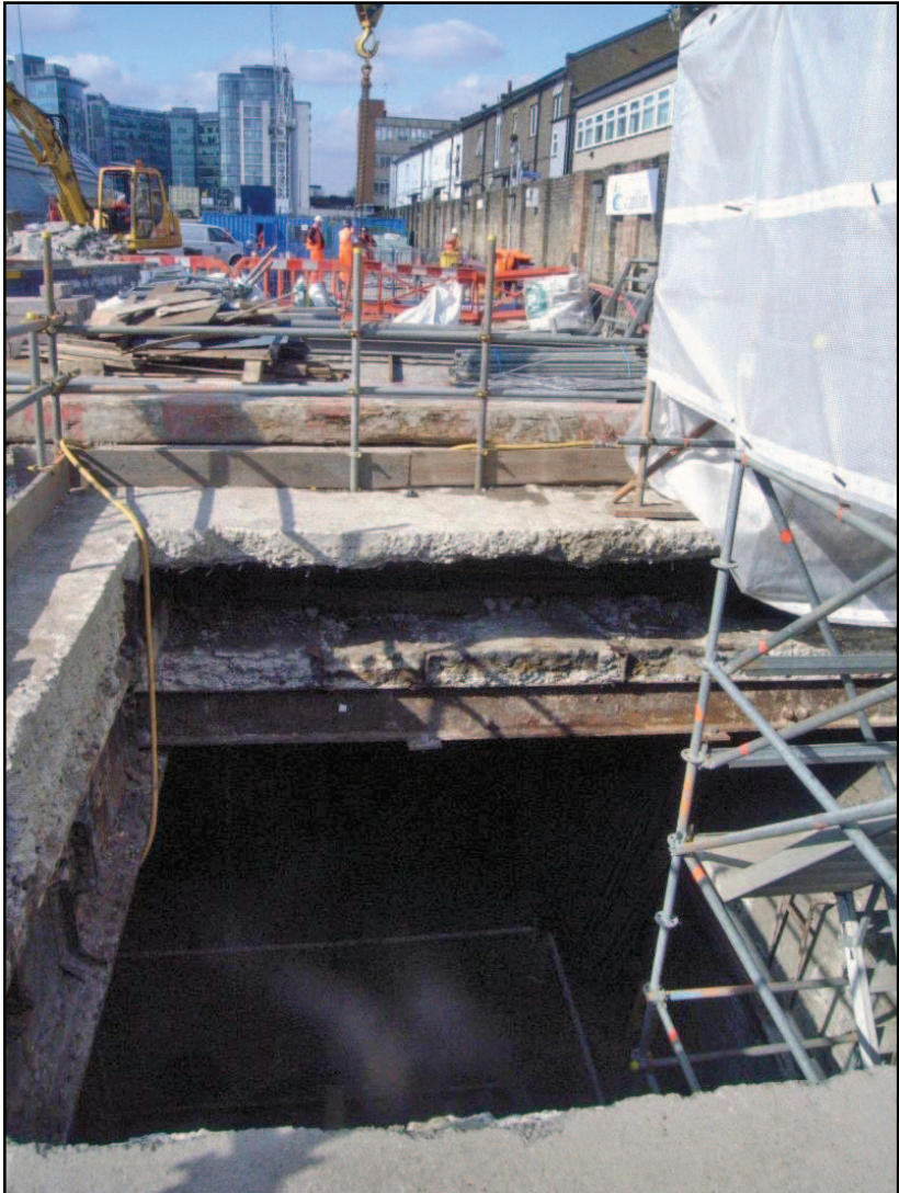
Plate 18: General View of the Upper Deck in the area of the Access Shaft
