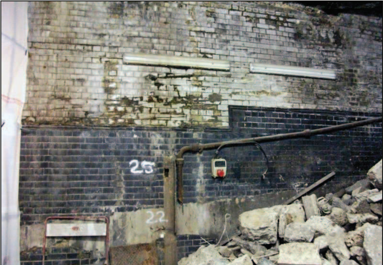
Plate 26: Lower section of Retaining Wall with scars of vehicle impacts
