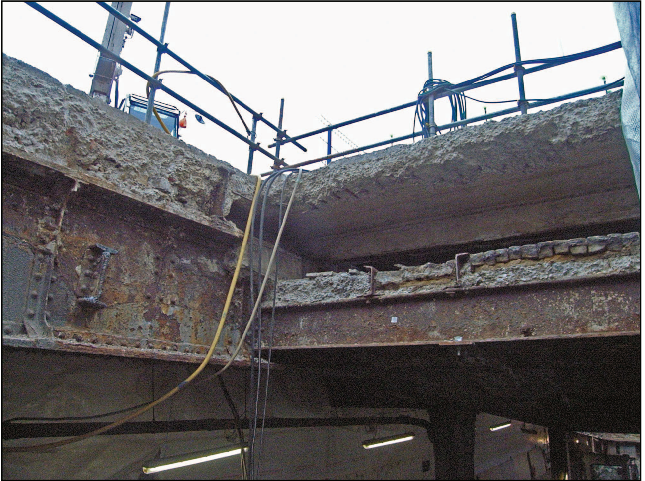
Plate 19: Section at the point where the Milk Ramp meets the London Street Upper Deck
