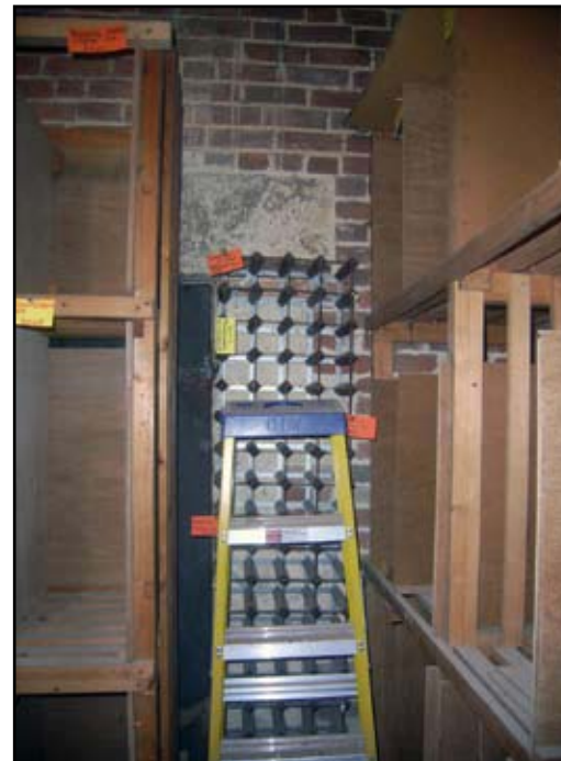
Plate 24: View of unused existing opening to Buttery Cellar in main Wine Cellar
