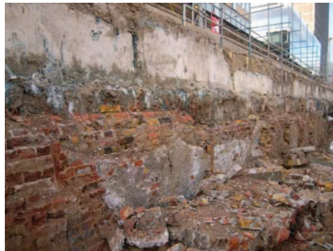
Second inner cellar wall added to inner face of original white washed southern wall of cellar (6546)
