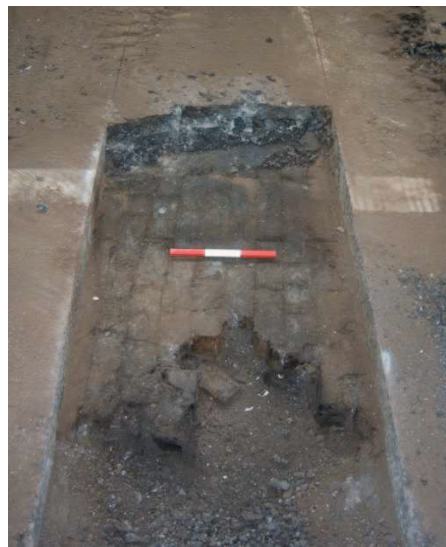
Decayed section of setts
