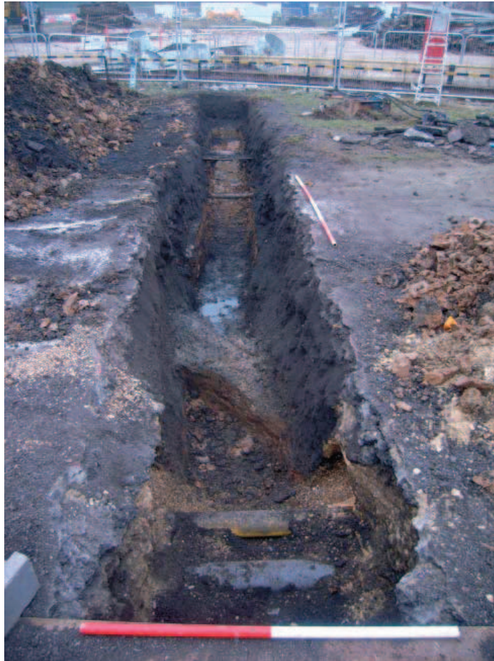
Plate 11: Trench 6. Southern end of trench looking north. Concrete encased water main [604] in foreground
