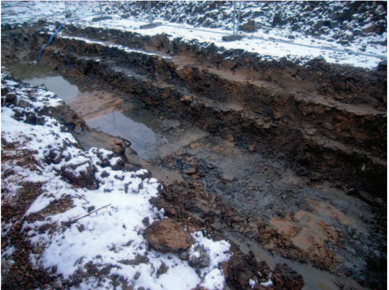
Plate 27: Trench 11. View of excavated trench looking W. Showing recent "madeground" deposit (1101) over Natural clay (1102)
