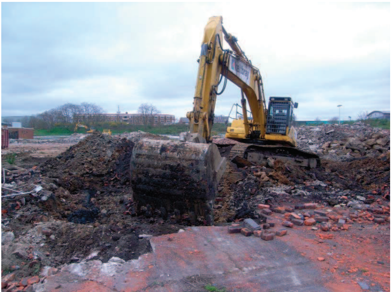
Plate 24: Trench 10. Concrete plinth [1002] for roof column of 1906 Engine Shed. Showing bolts for column and central hole for vertical down drain pipe
