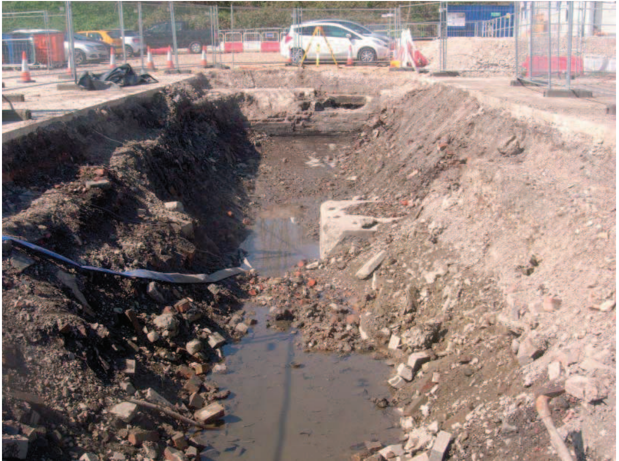
Plate 43: Trench 12. Overview of trench from E. Showing pivot base [1203] turntable floor (1223) and W turntable sidewall [1235]
