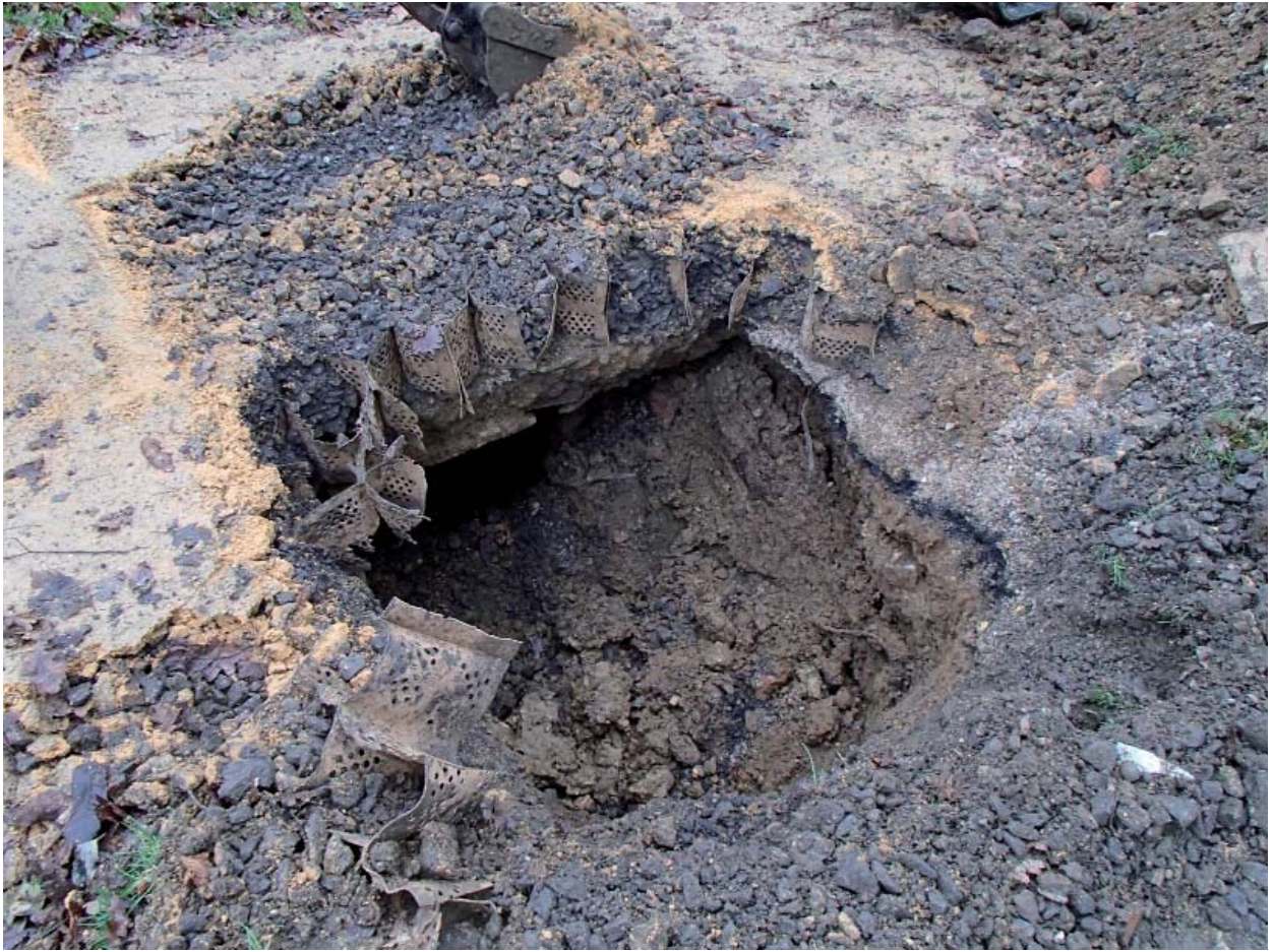
Plate 1: Showing collapse of path
