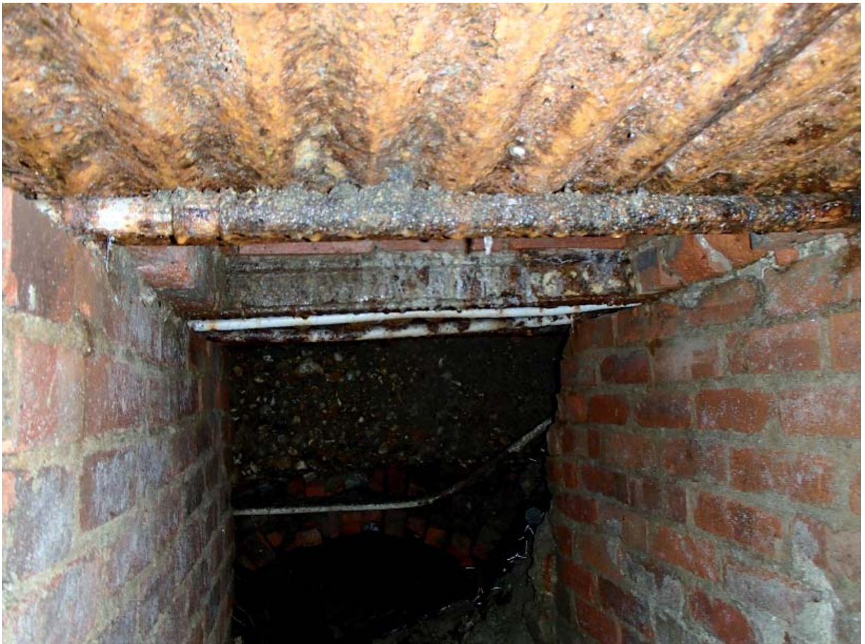
Plate 2: State of corroded concrete slab
