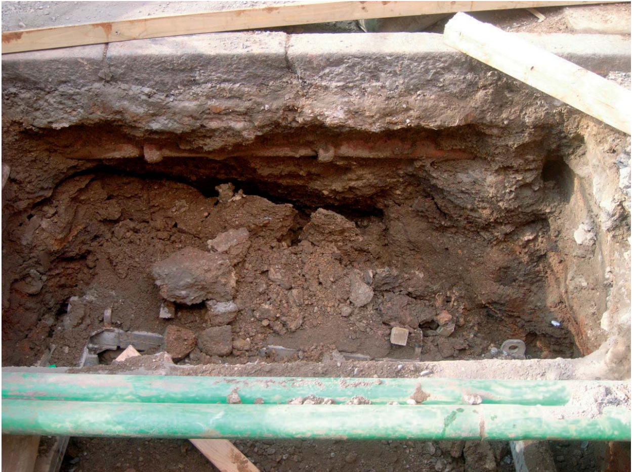
Plate 7. West section, showing collapsed deposits on removal of the shuttering, looking west
