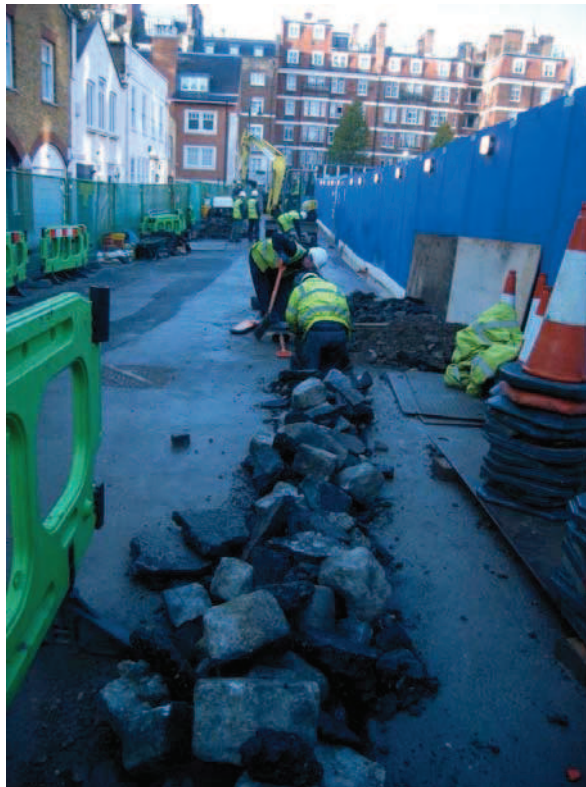
Plate 3: St. Anselm's Place, a third service diversion trench being dug, the earlier ones are to the left of the picture, looking west.
