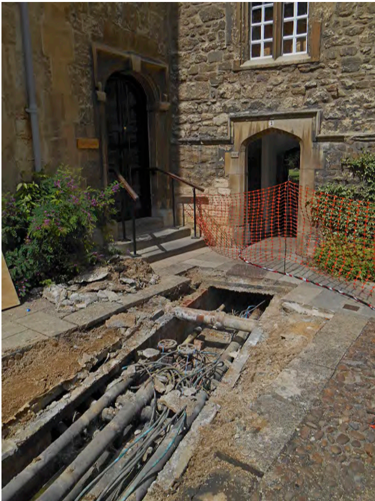
Plate 4: Area on the west side of the Quad, showing the brick lined cable duct
