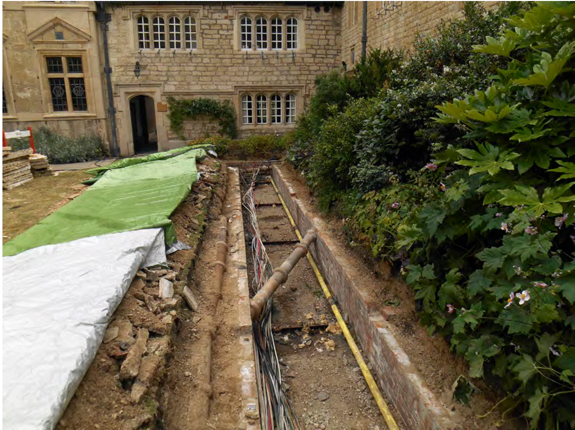
Plate 3: Area on the south side of the Quad, showing the brick lined cable duct
