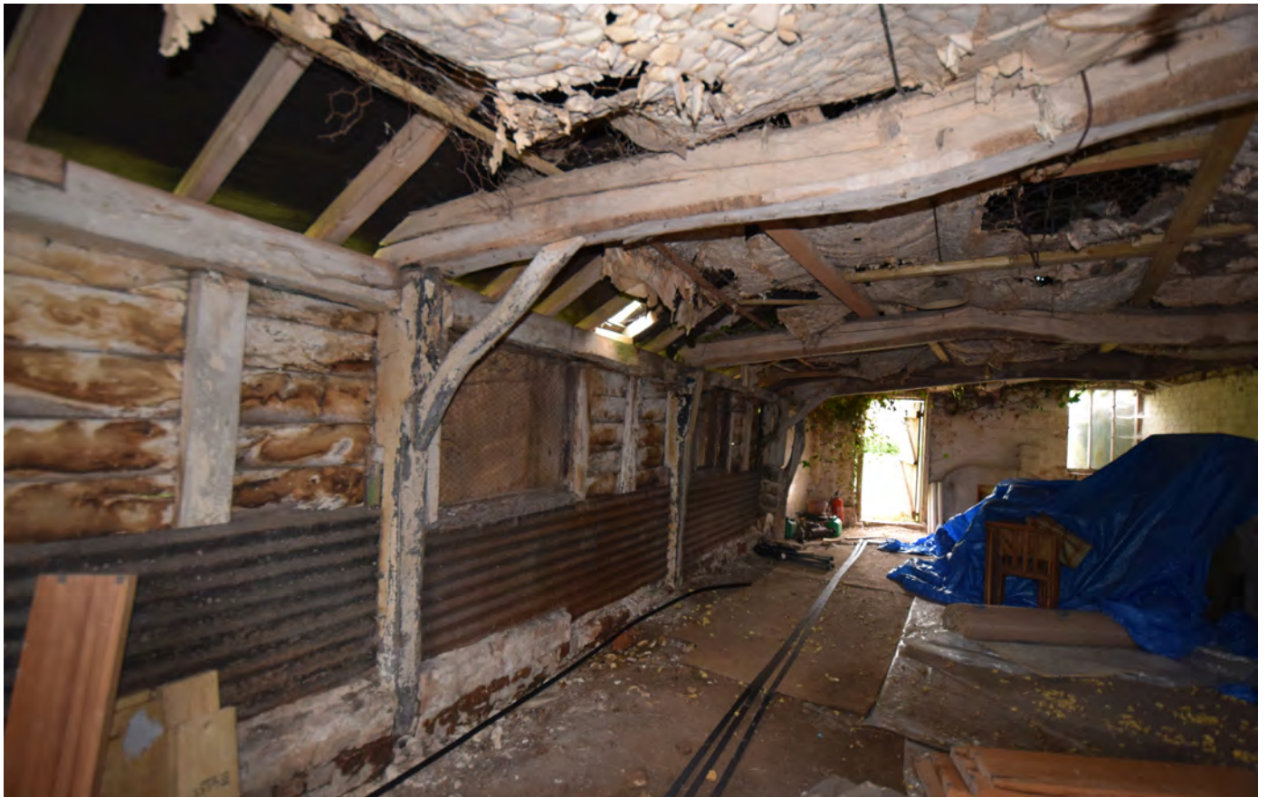
Plate 12: The north wall of the north half of the barn, before stripping
