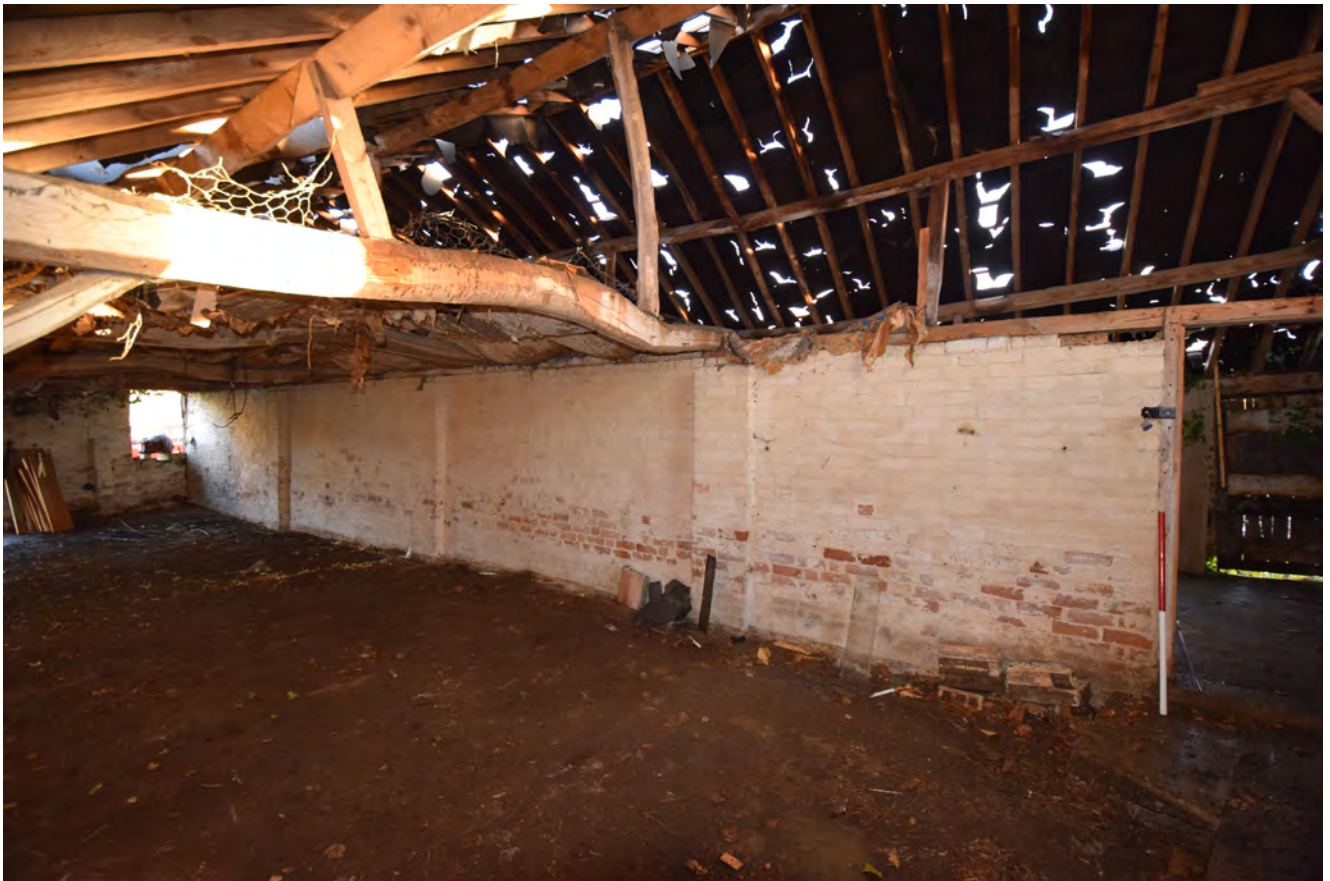
Plate 10: The brick wall along the centre of the barn. Looking south east
