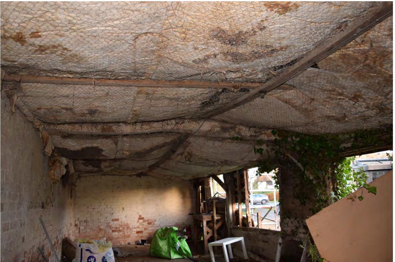
Plate 14: The 'ceiling' of the barn. South half of the bar, looking east
