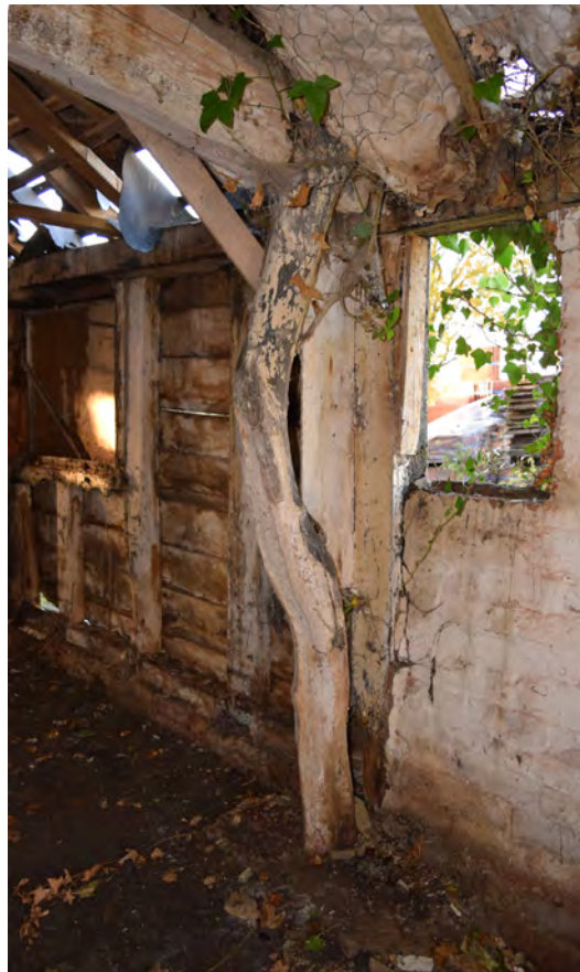
Plate 18: Irregular timber brace. Easternmost bay, north half of the barn
