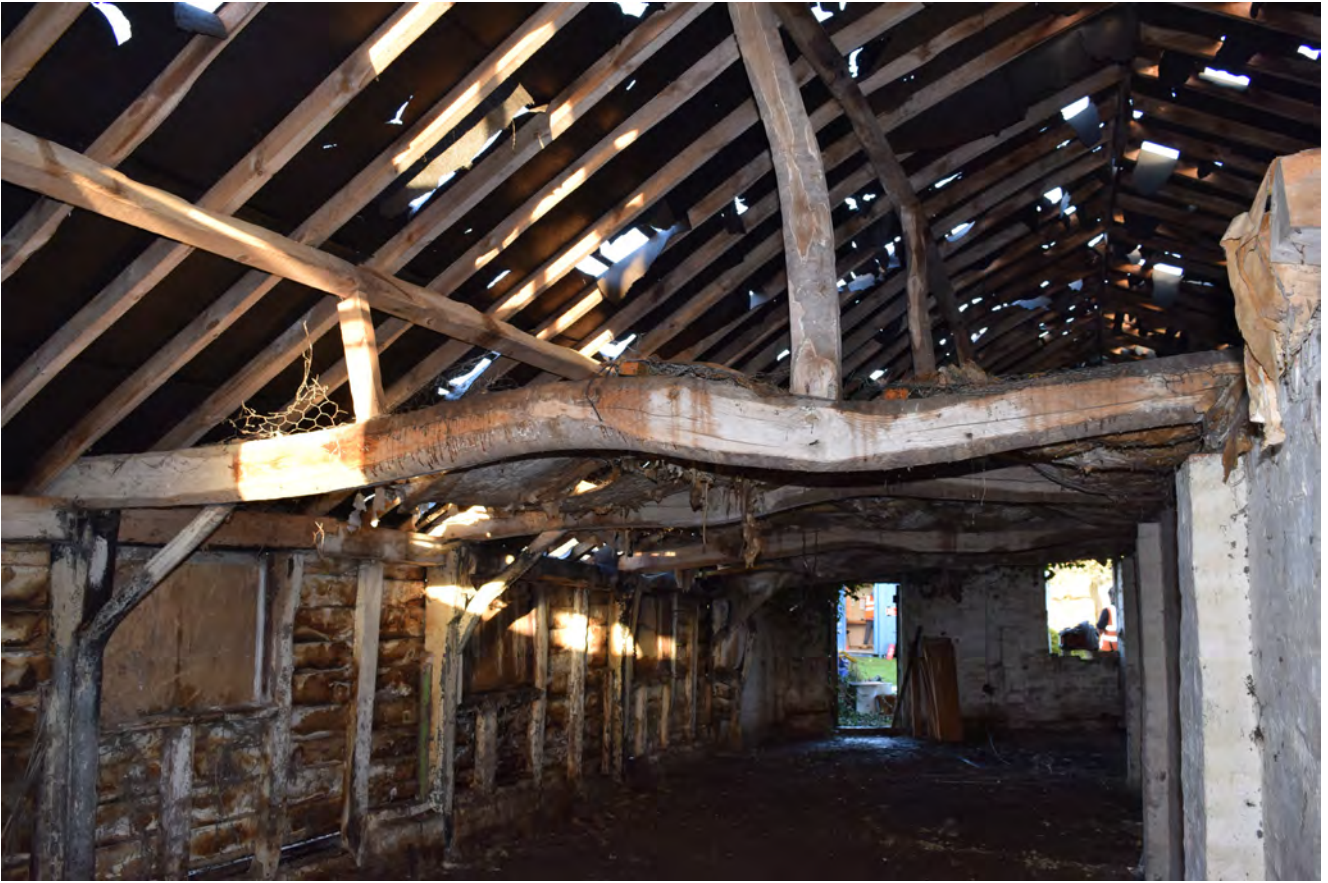
Plate 15: The later roof structure, viewed over the 'ceiling'. North half of the barn, looking east
