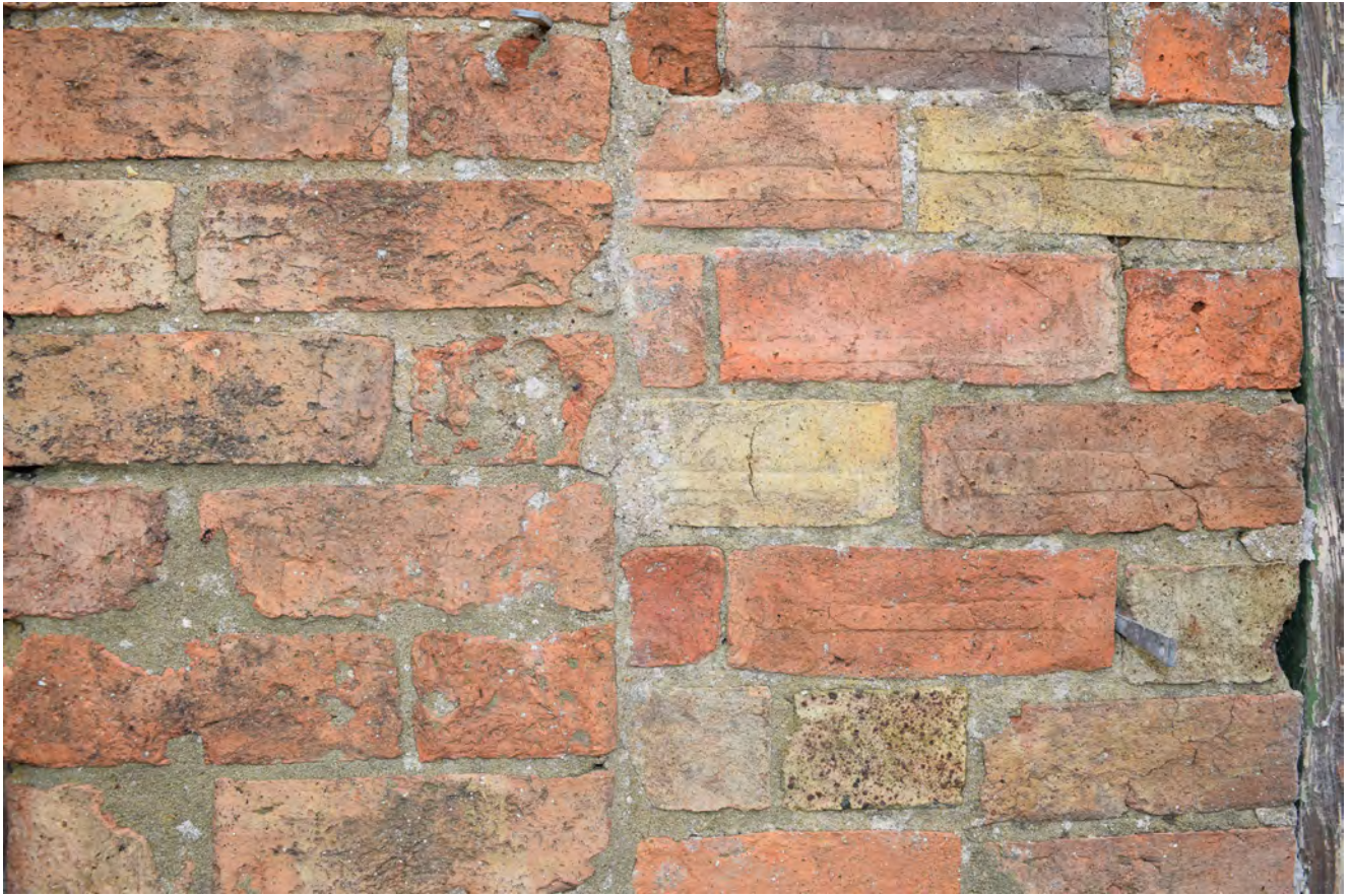
Plate 23: The bricks of the east wall of the barn and the repair of the lean-to. Looking north
