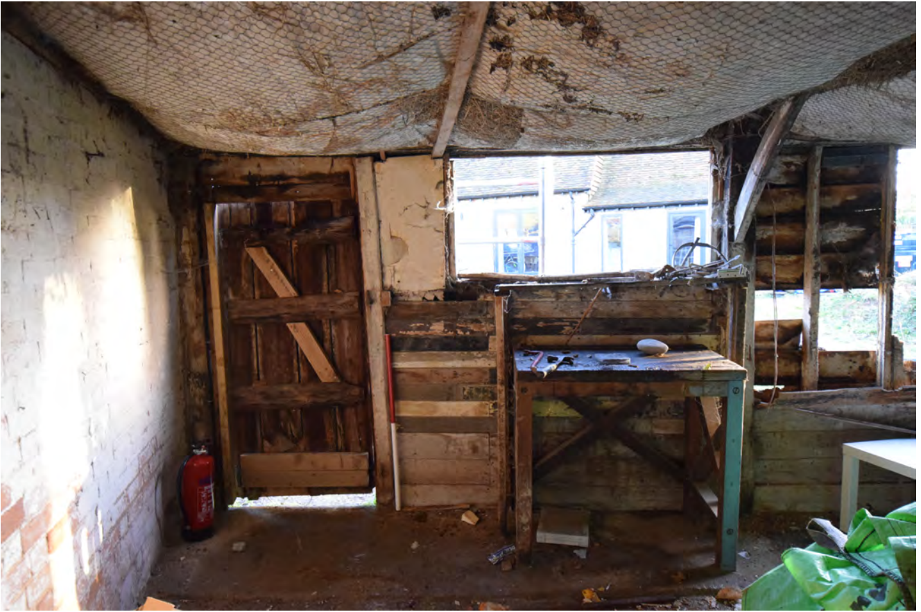
Plate 13: The south wall of the east bay of the barn. Looking south
