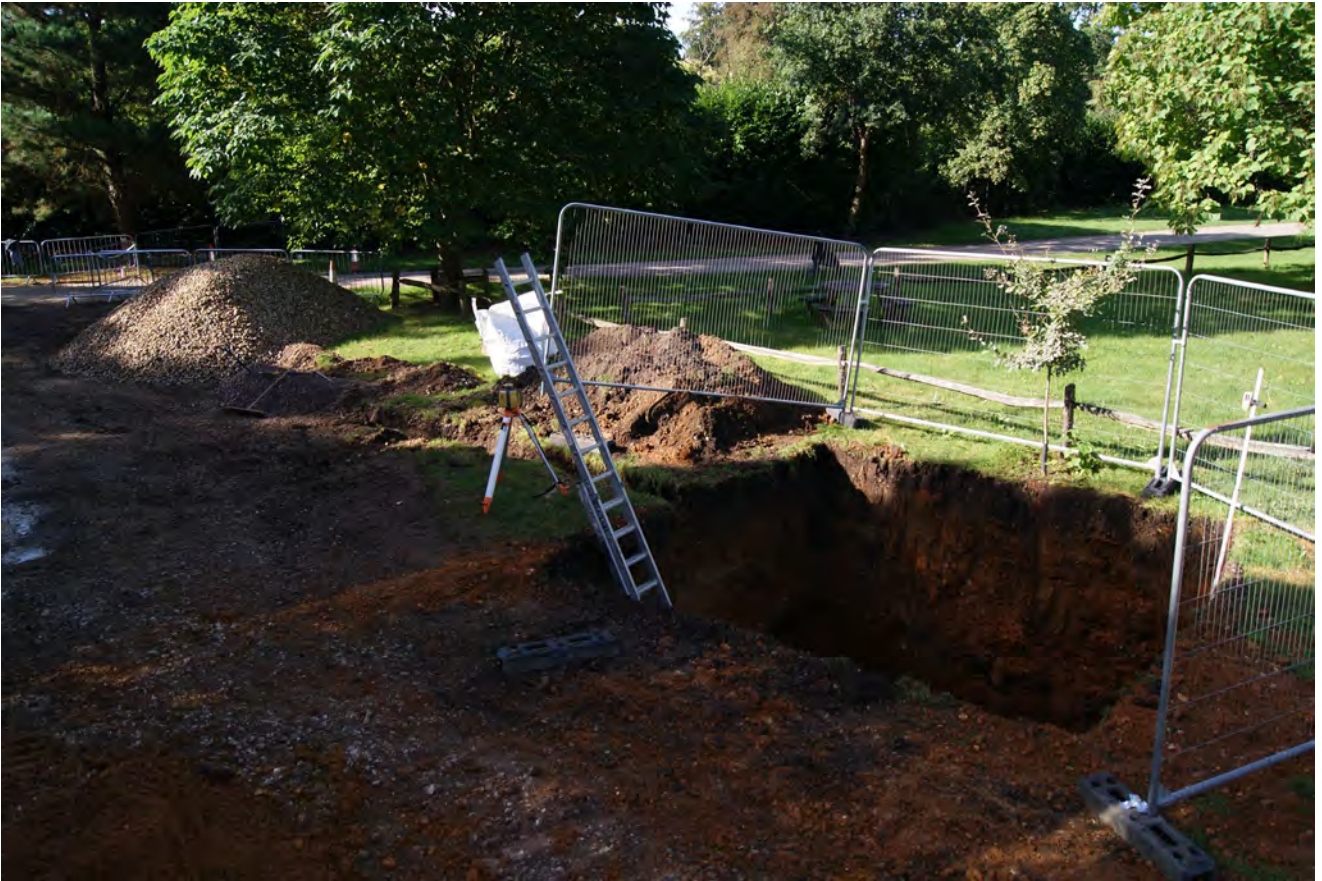
Plate 12: General view of soakaway hole (c.35 m to N of S end of trench), looking south west
