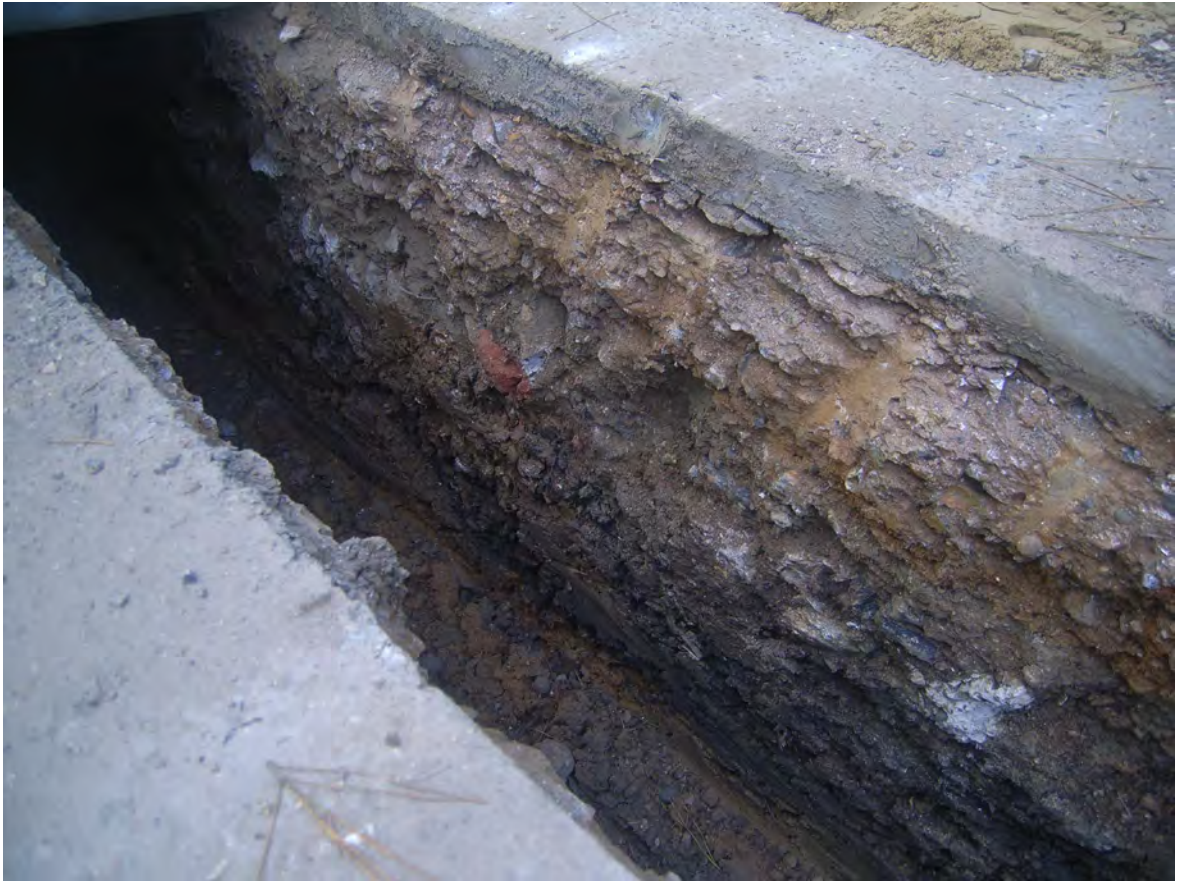
Plate 6: Side of trench where it crosses road at S end of car park, looking south west
