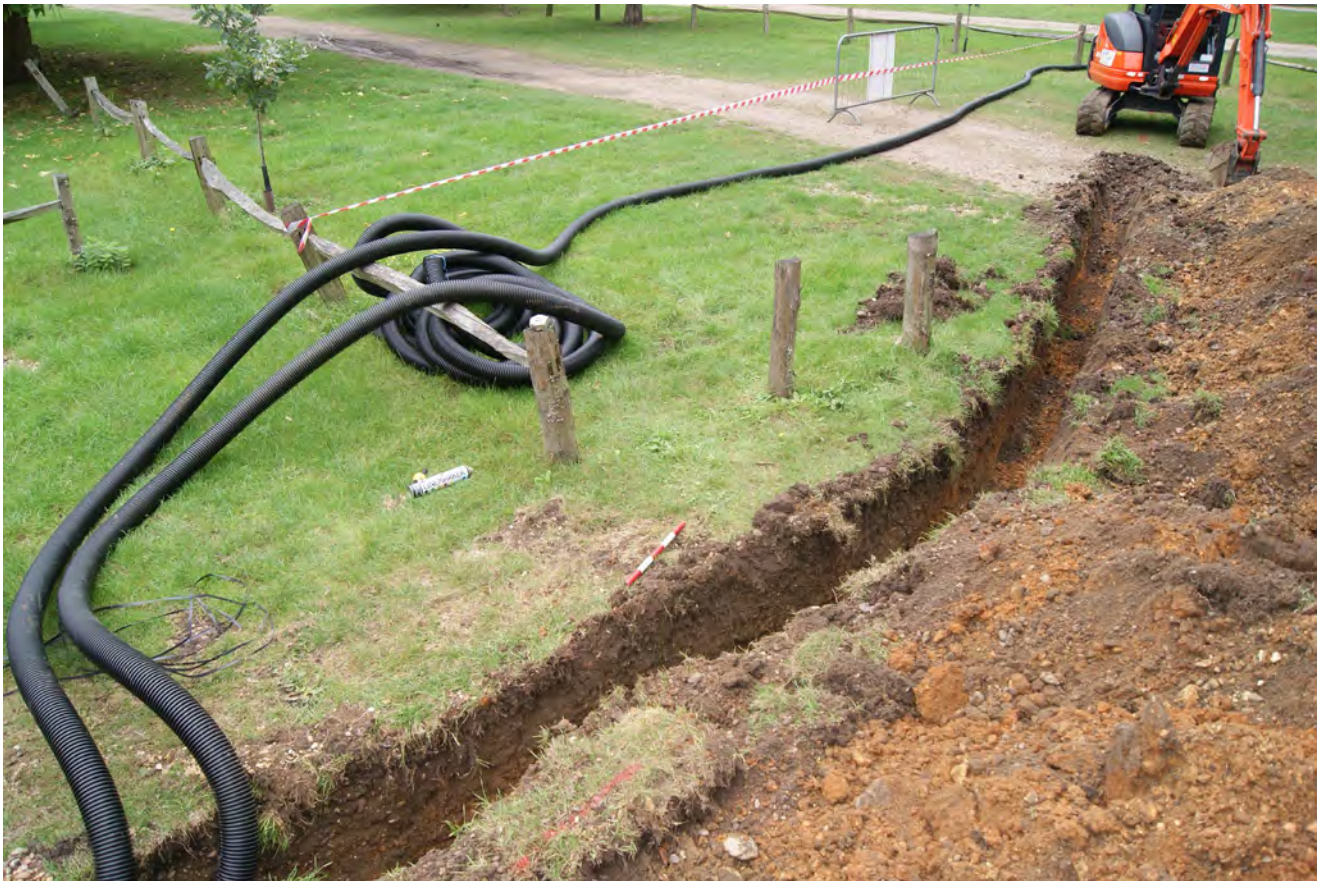
Plate 9: Trench towards centre of car park (c.50 m N of S end), looking north
