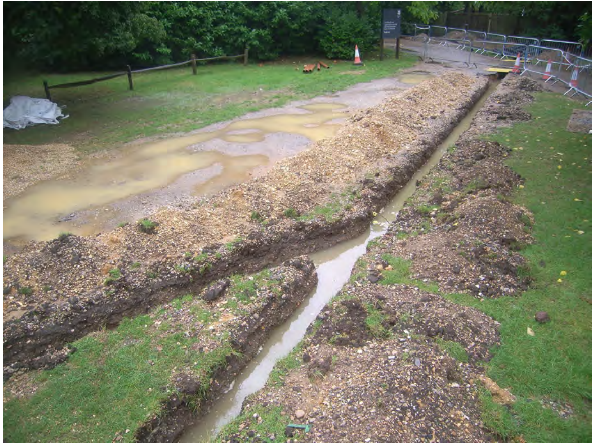
Plate 8: Section of trench immediately N of road in car park, looking south
