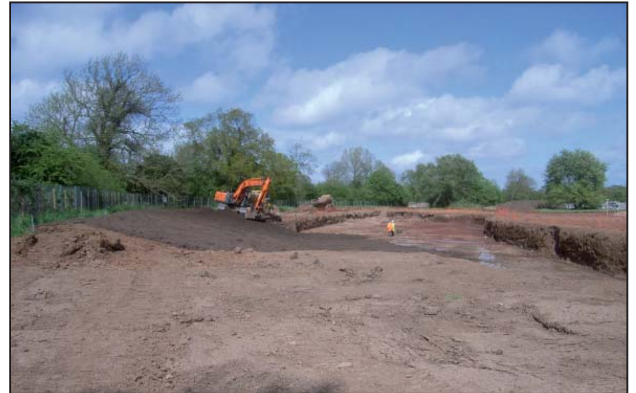
Plate 4: West Field, reduction of the area to form the Balancing Pond, looking north
