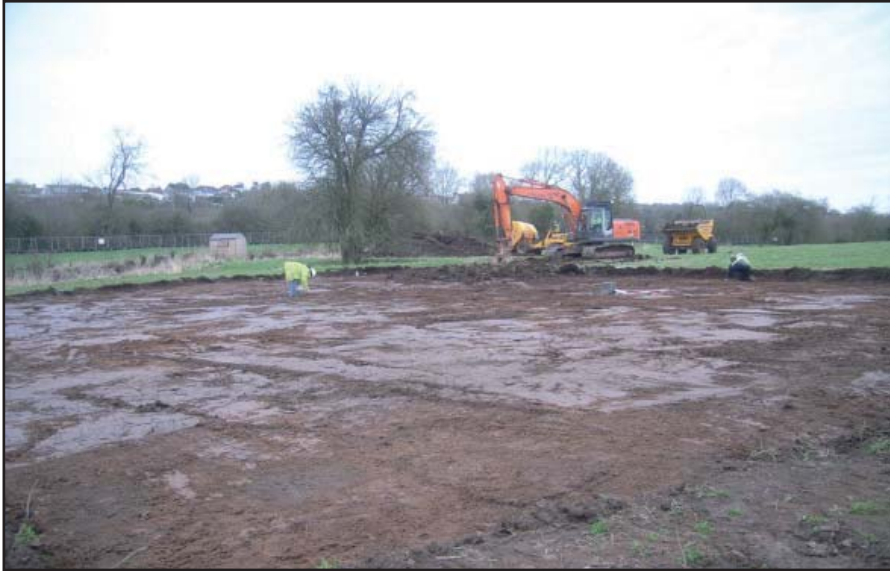
Plate 1: Main Field, laydown area, stripping by 360o excavator being supervised, looking north
