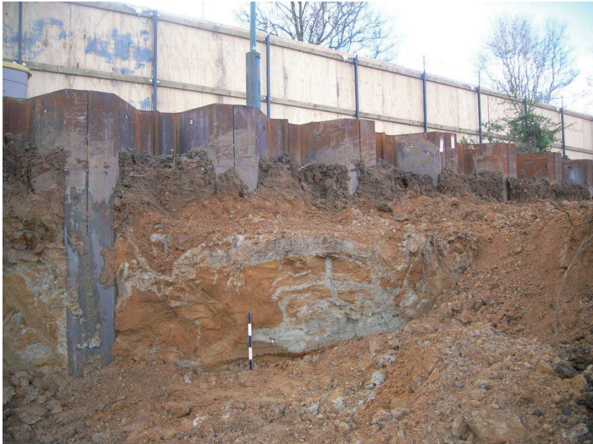
Plate 4: Section revealed by the sheet piling works along the Site's western edge
