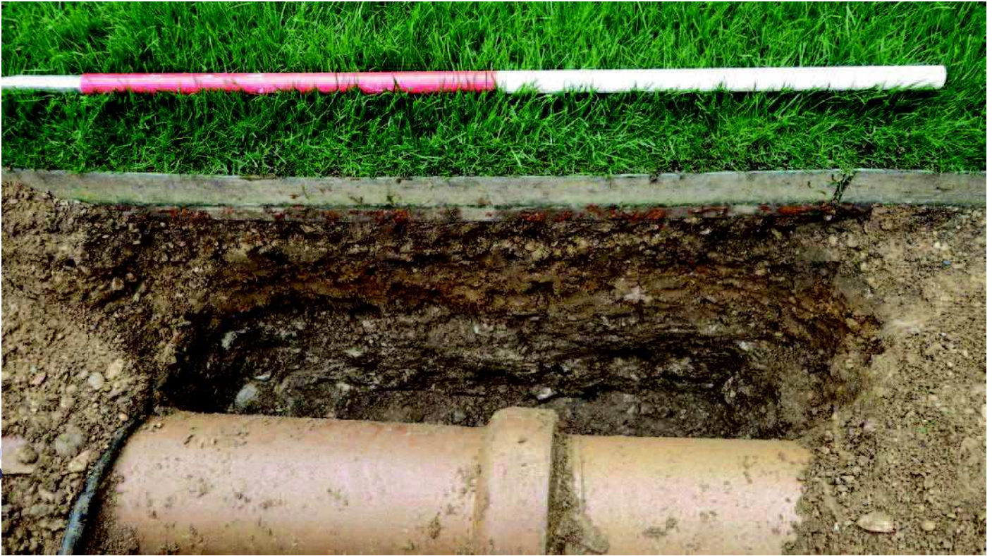
Plate 7: Section 6, Base of bank in north Main Quad, looking north
