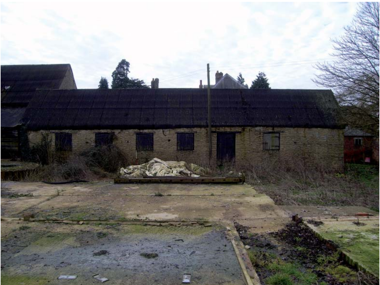
Plate 4: Stable or loosebox to the west of the threshing barn; north elevation
