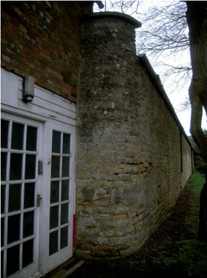
Plate 43: Barns 4 & 5; join between the block and the farmhouse on the south elevation
