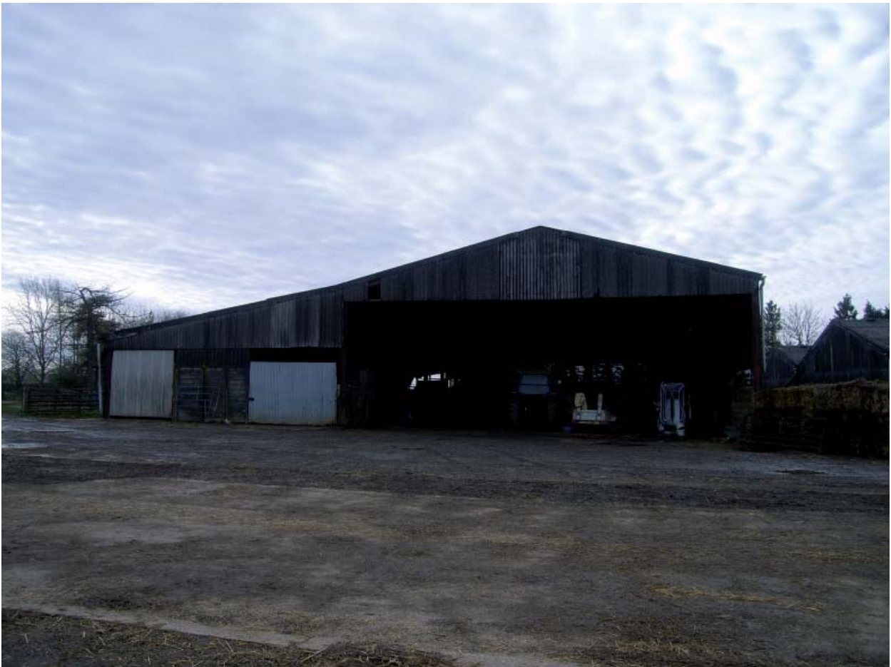
Plate 6: Modern building to the far eastern end of the site; north elevation
