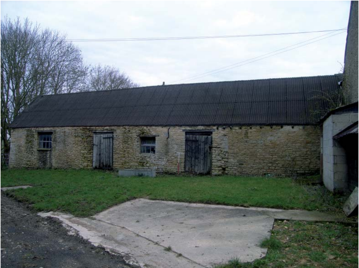
Plate 3: Stable or loosebox to the west of the threshing barn; south elevation
