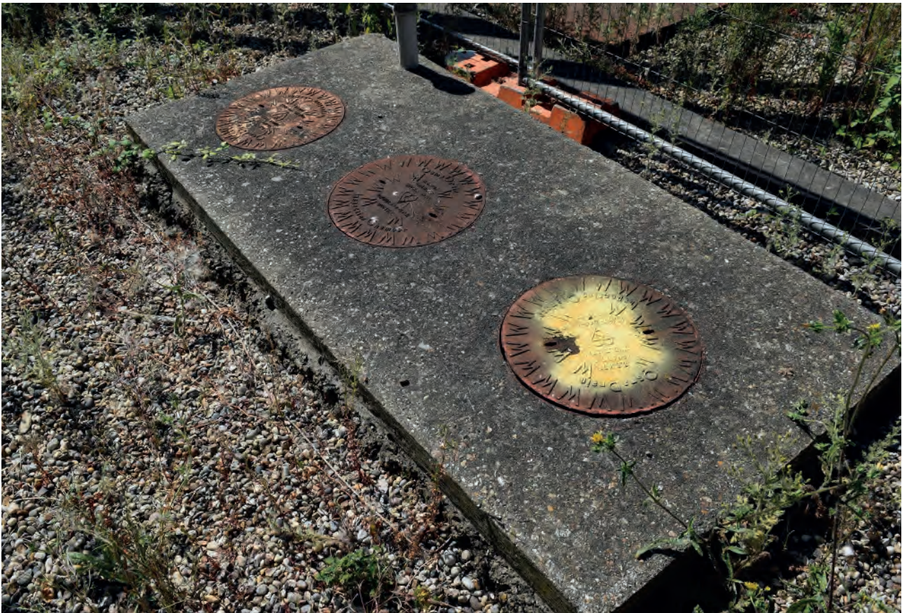
Plate 90: Drainage 'separator' between holders
