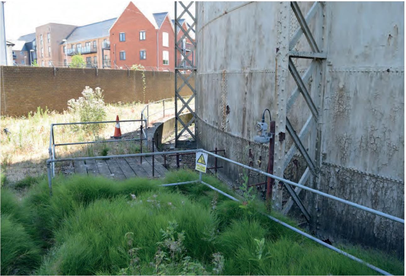
Plate 11: Valve Pit to north side of 114
