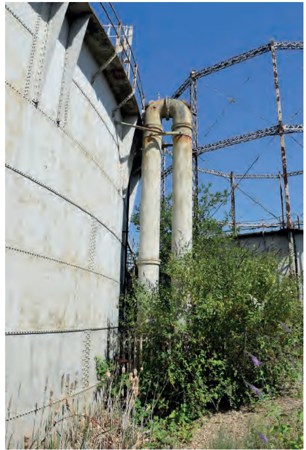
Plate 66: Anti-flooding pipes to east of Holder 115
