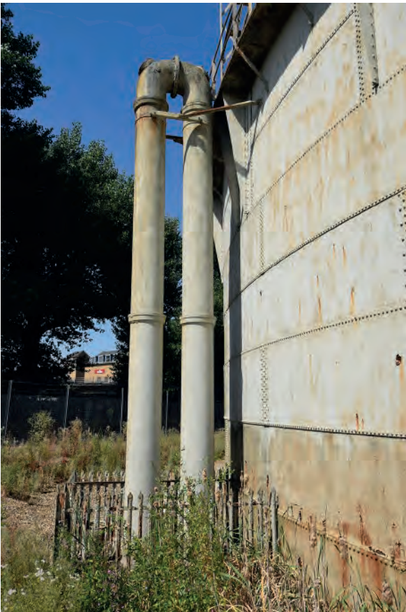
Plate 67: Anti-flooding pipes to east of Holder 115
