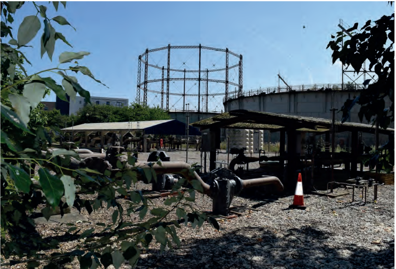
Plate 80: Plant in Pressure Reduction Station to NW of 115
