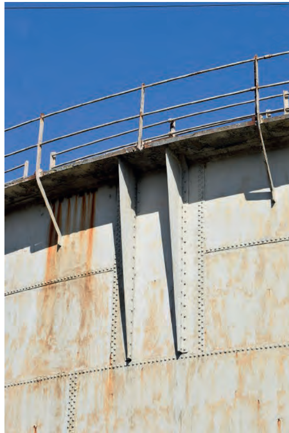
Plate 64: Detail of support brackets to Holder 115
