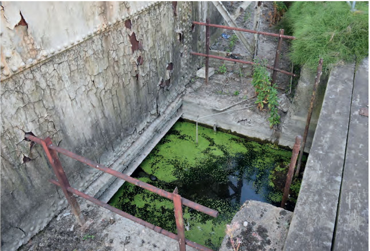
Plate 12: Valve Pit to north side of 114
