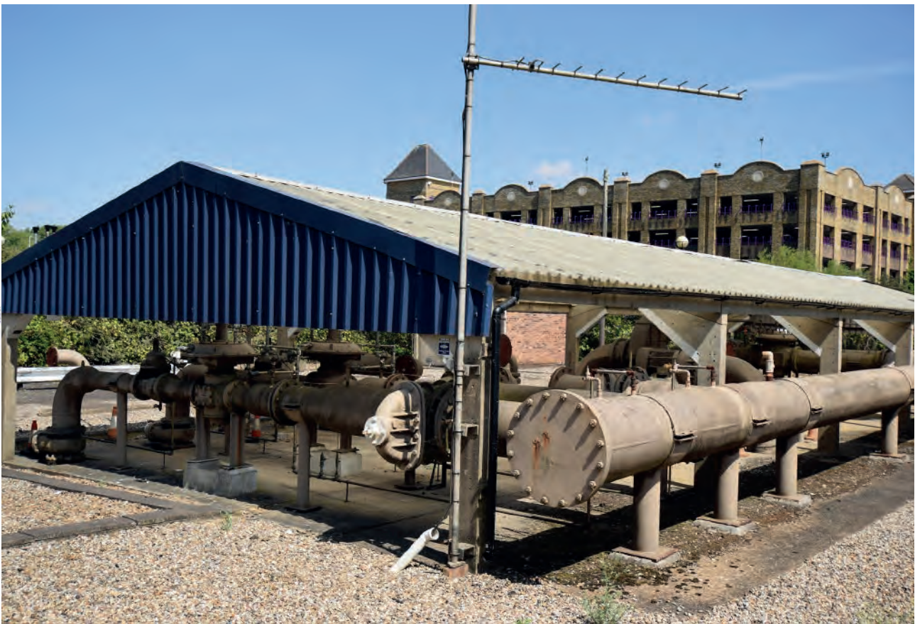
Plate 89: Plant in Pressure Reduction Station (still operational)
