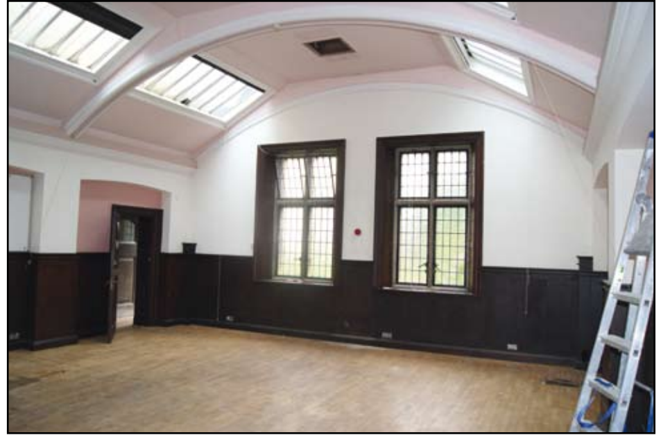
Plate 34: West wall of former lecture room
