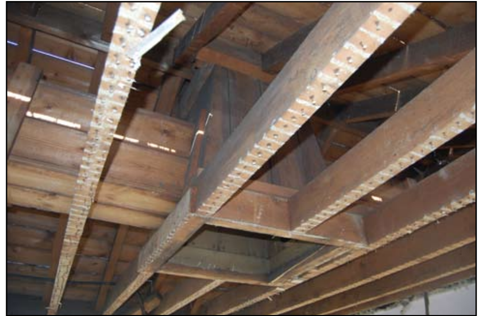
Plate 46: Duct in ceiling
