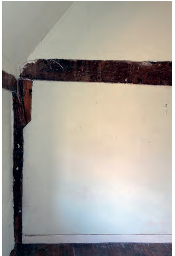
Plate 141: The post and tie beam at the east end of the south wall in bedroom 6
