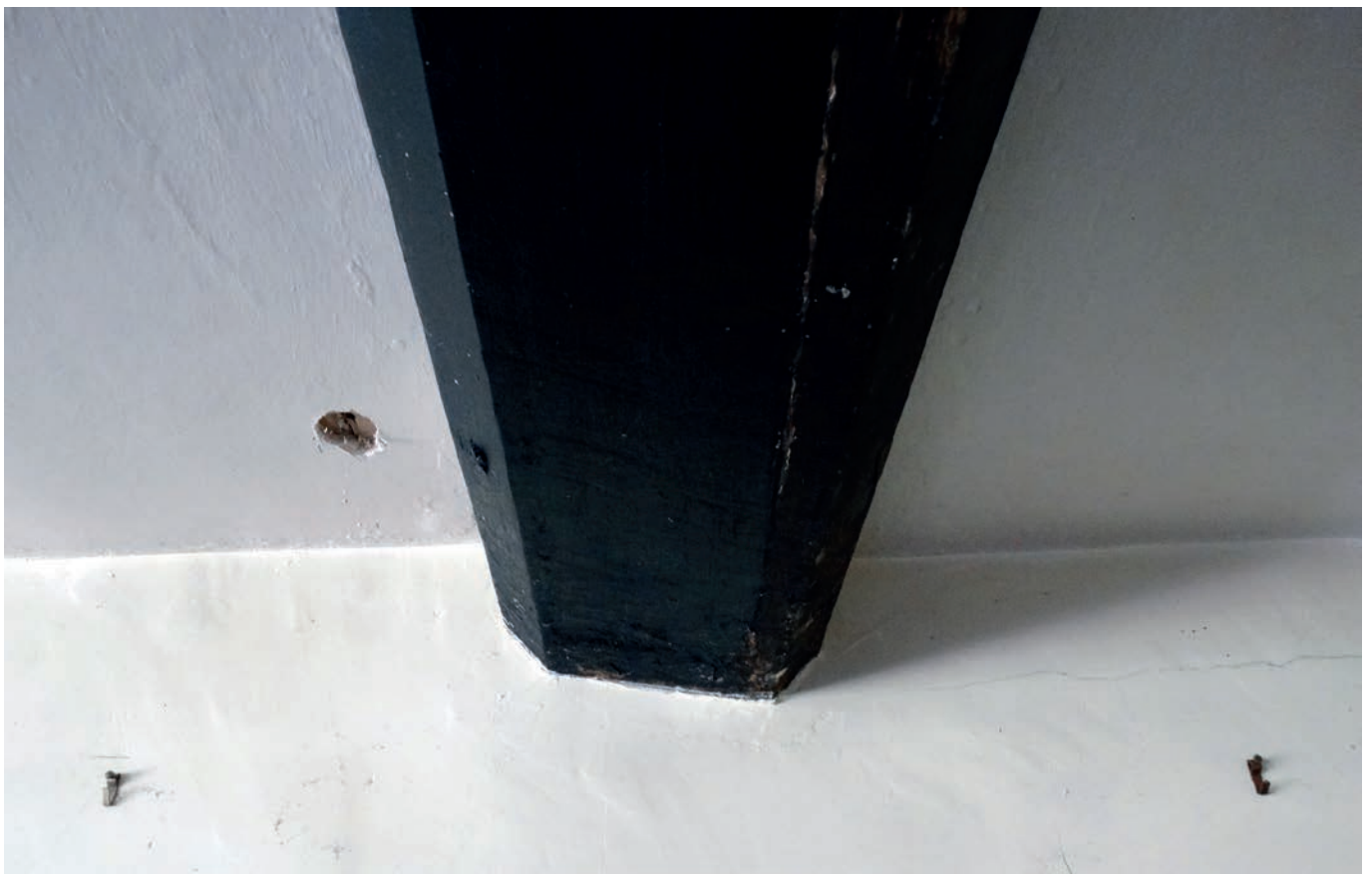
Plate 70: The chamfered beam in sitting room 2, the stop being in the later pantry
