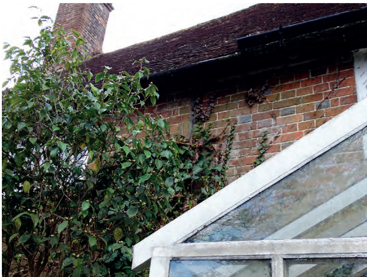
Plate 11: The join in the brick façades of the central and north bays
