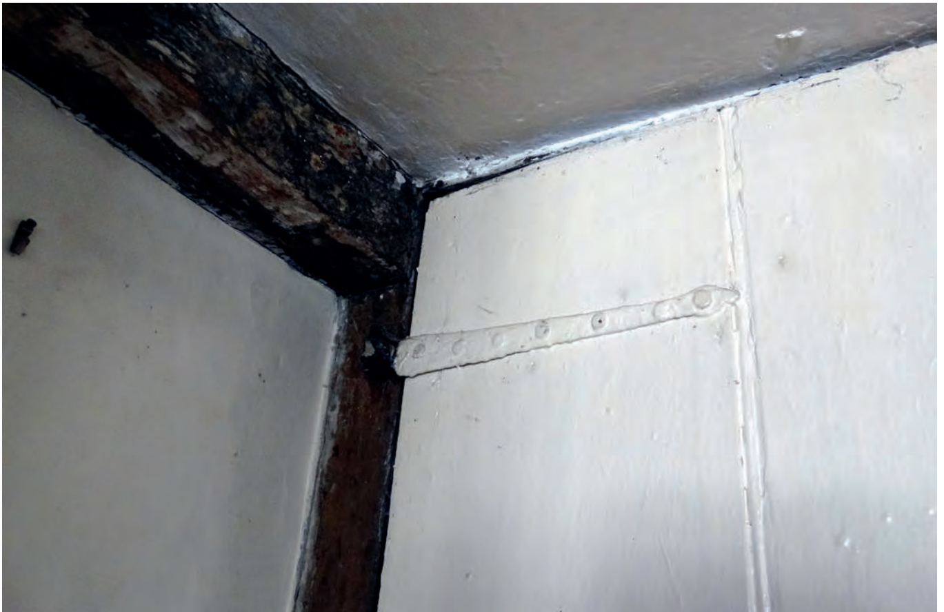
Plate 74: The strap hinge to the door between sitting room 2 and the southernmost staircase
