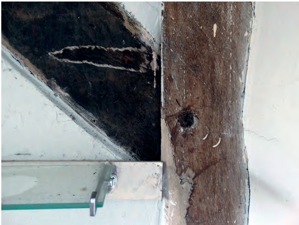
Plate 135: The carpenter's marks between the post and brace at the east end of the frame
