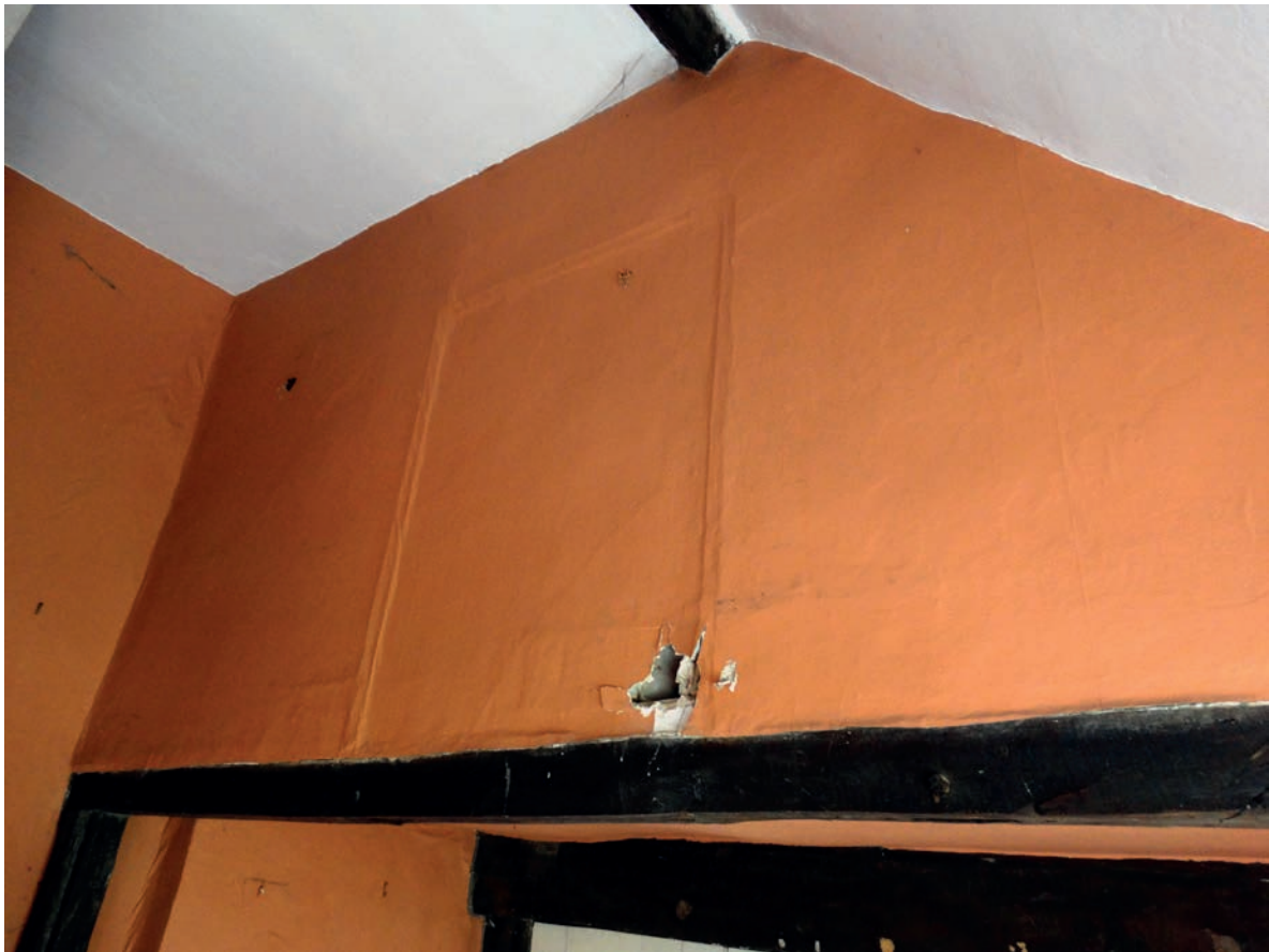
Plate 123: The blocked up water tank cupboard in bedroom 5
