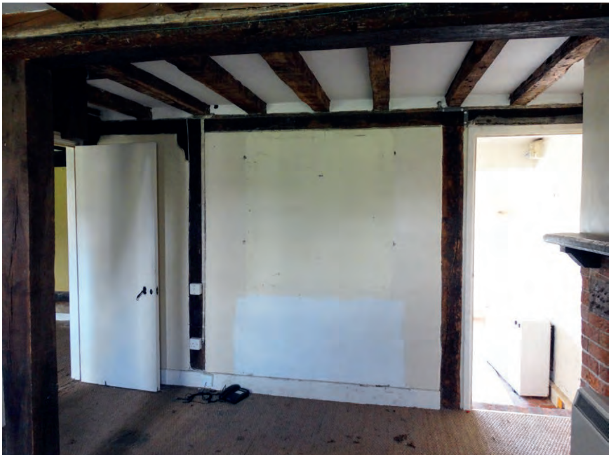
Plate 25: The timber frame visible in the west wall of the entrance hall
