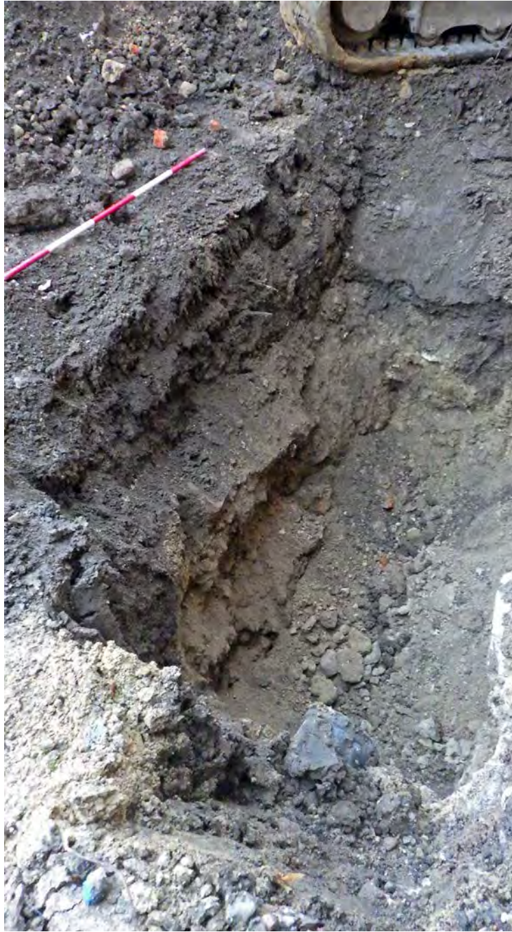
Plate 13: Chavasse Quad, section of test pit to investigate the foundations of the north wall of New Road Baptist Church, facing north-east
