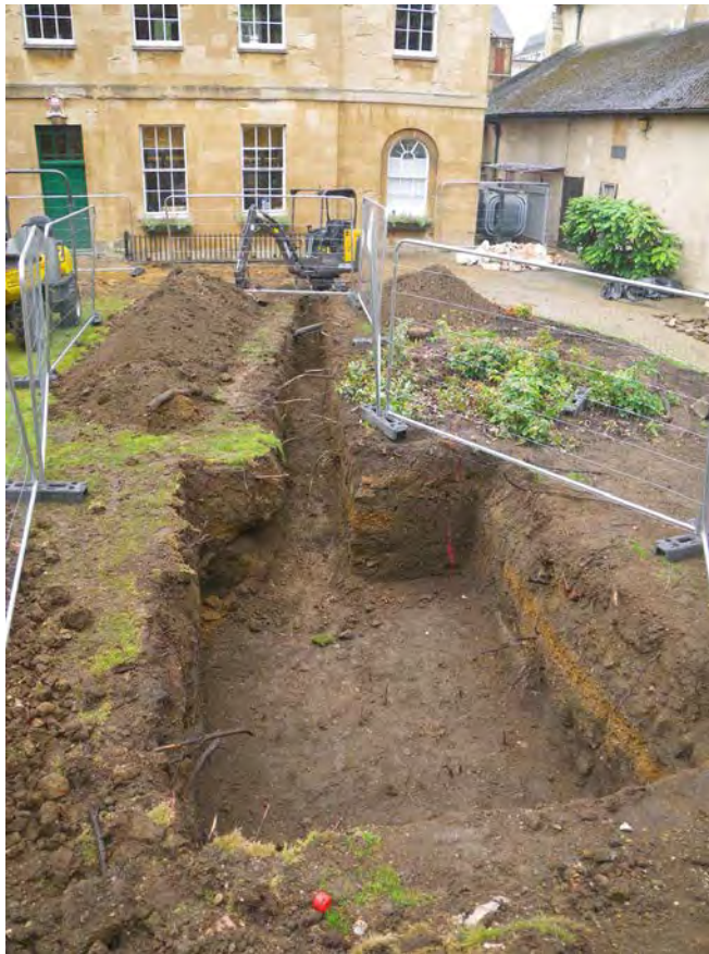
Plate 3: Linton Quad watching brief, soakaway and service run general shot, facing east
