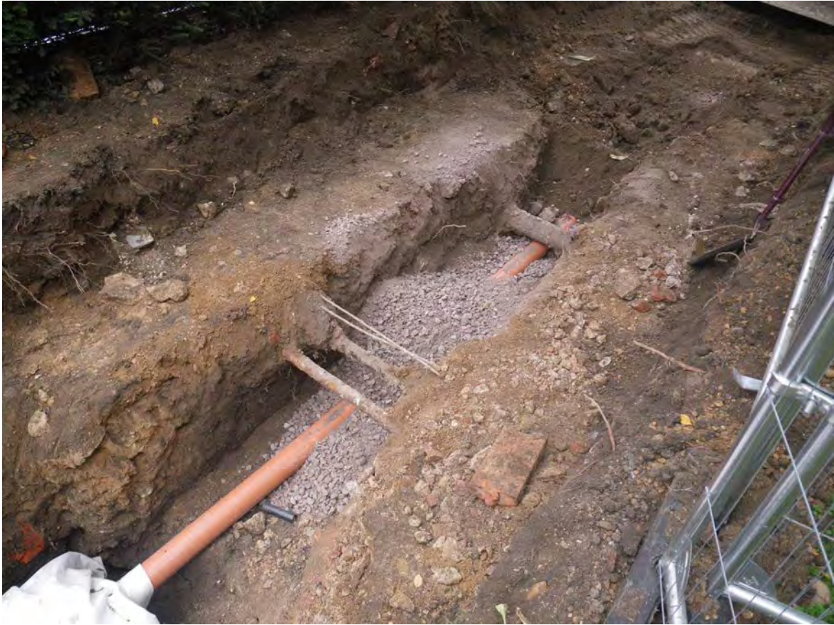
Plate 5: Linton Quad watching brief, new water pipe and previous services in the service trench on the New Inn Hall Street frontage, facing north
