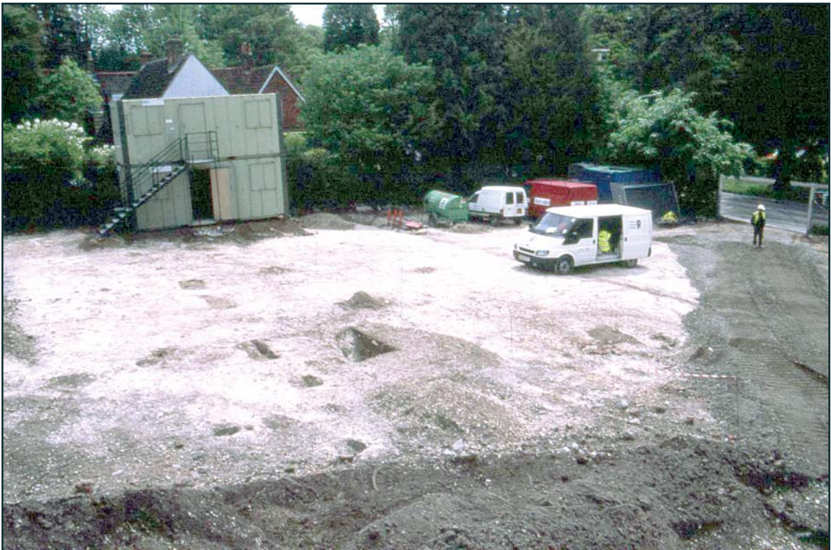
Plate 2: Looking south-west across south of site, Fence line 1 in the centre, running towards the portacabins
